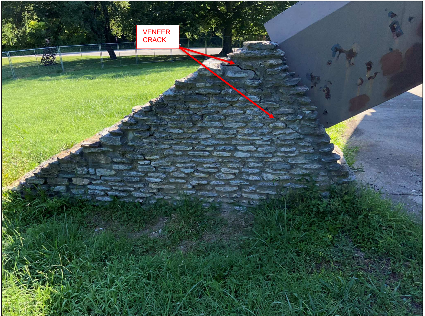
Photo 2: Abutment #8 Veneer Cracks
