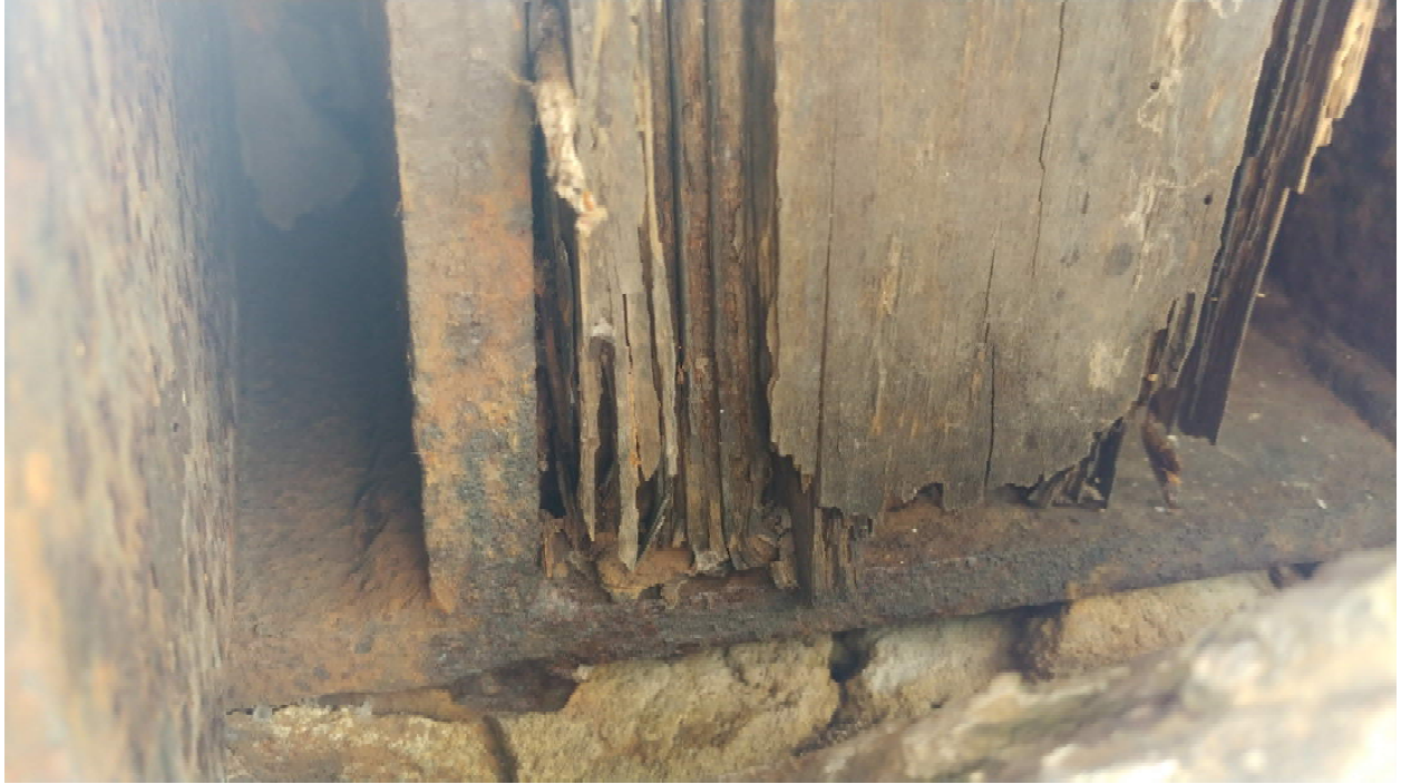
Photo 1 – Wood rot and decay at base of glulam arch.
