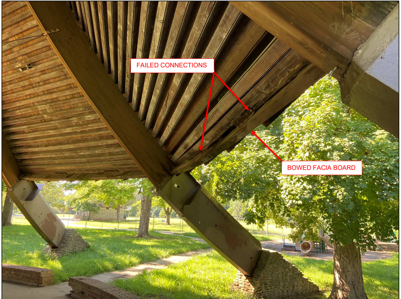
Photo 7: Bowed Fascia Board
