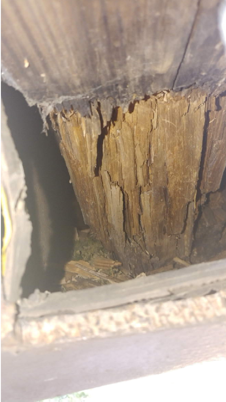
Photo 4 – Glulam arch wood deterioration near the top of the steel casing.
