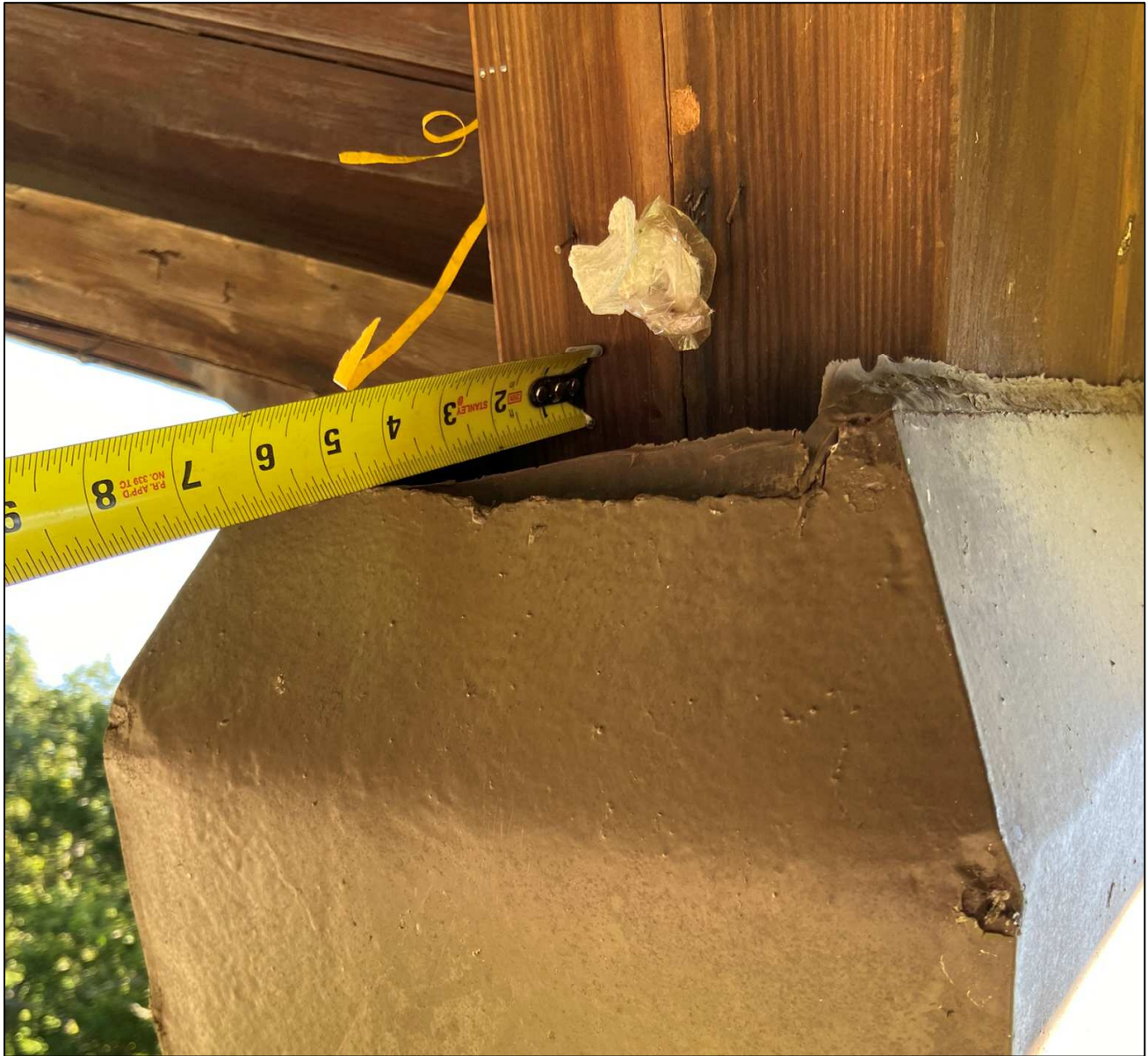
Photo 4: Measured Gap at Beam #6
