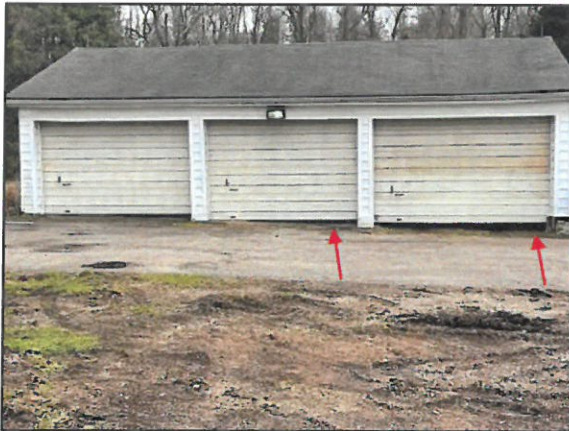
PHOTO NO. 11: Ground subsidence at garage
