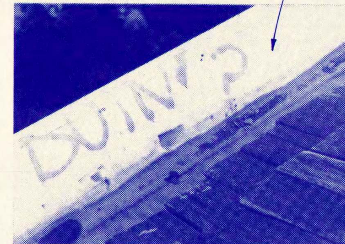
REMOVE ALL NAILS AND ASPHALT SHINGLES WHERE SHAKES AND GUTTER LINER ARE TO BE INSTALLED
