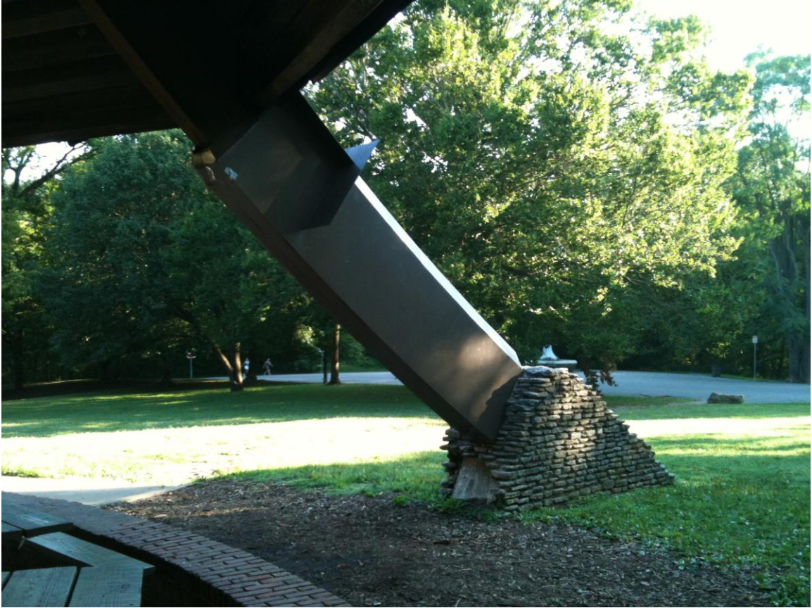
Steel sheath encasing the laminate beams from the buttress to the fascia board
