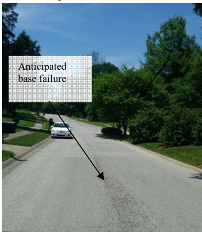
Photo #11: Northbound lane looking southwest at 407 Lake Forest Pkwy (to be regular asphalt)
