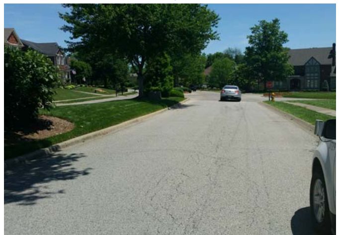
Photo #16: Northbound Lane Looking northeast to Woodlake Dr (to be regular asphalt)
