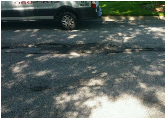
Photo #3: Base failure observed in southbound lane between photos 1 & 2
