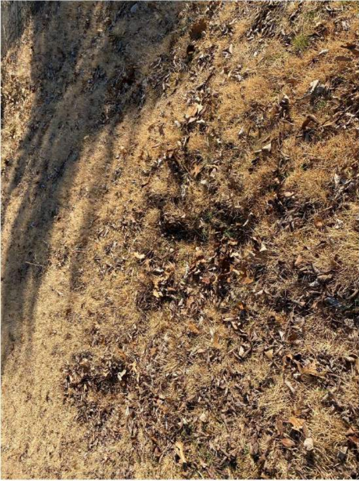
Feature 20- Possible Erosion
