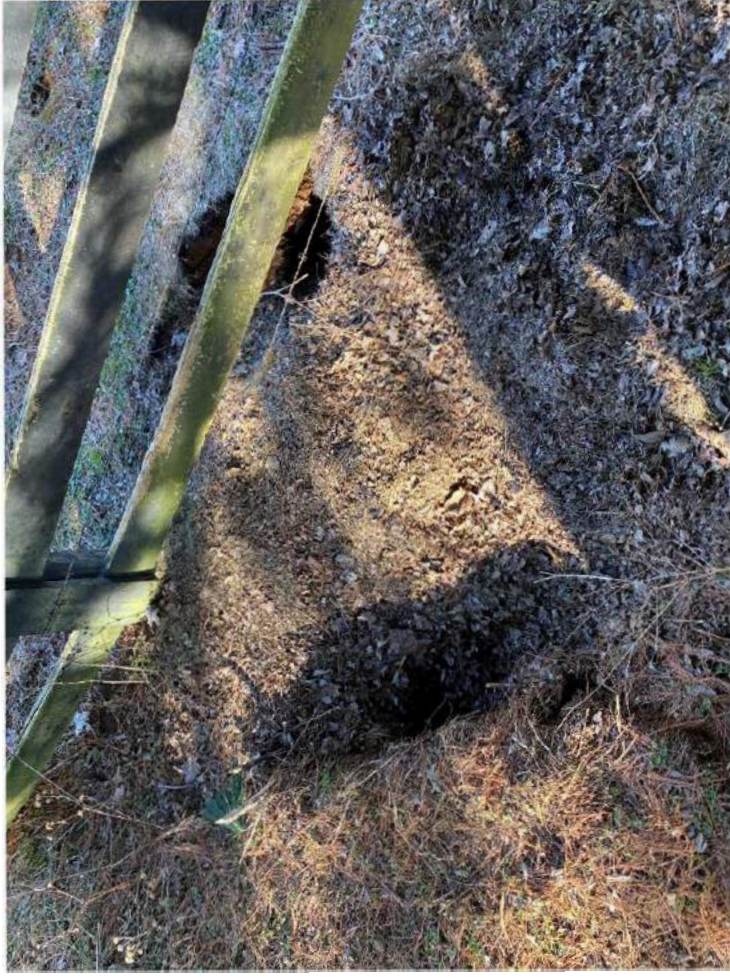
Feature 15- Possible Erosion
