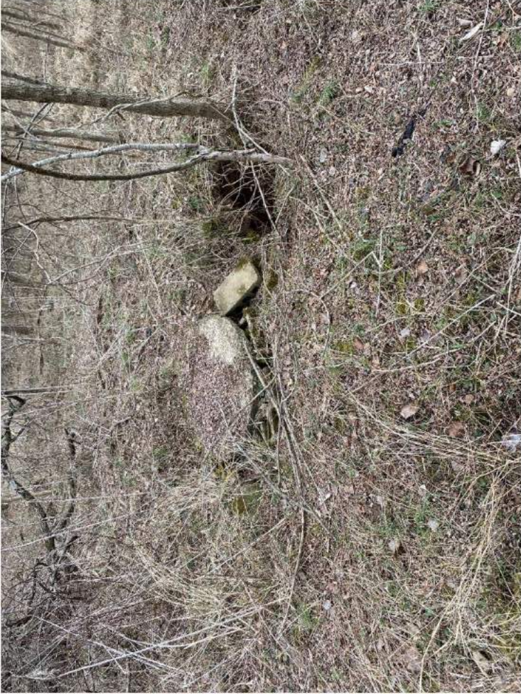
Feature 3- Erosion Features with Manhole Cover
