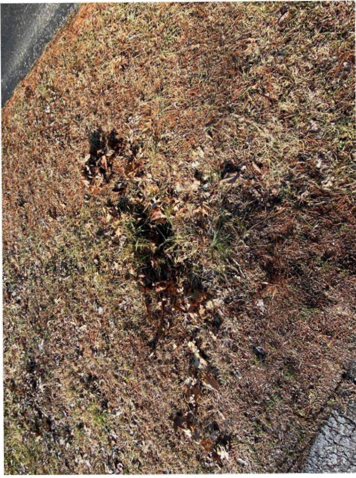
Feature 22- Erosion Throat
