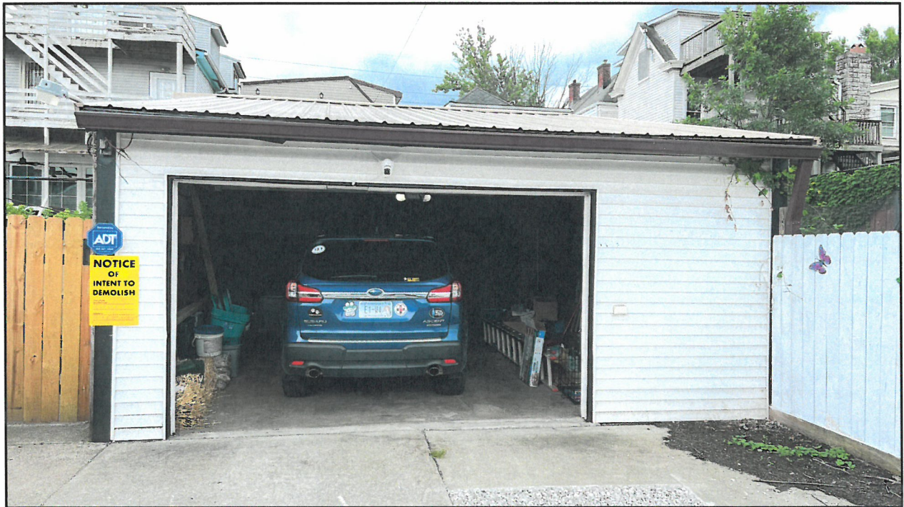
Current from public alley - Existing garage right side has 0' setback This garage will be torn down.
