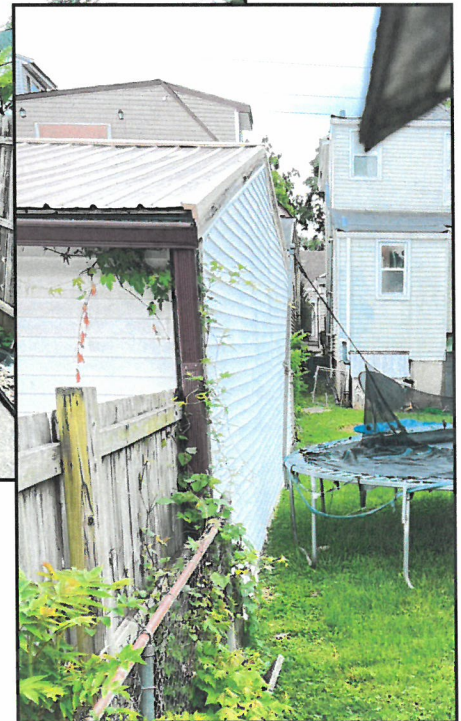
Existing view from property line on alley side showing existing setback of 0'.
