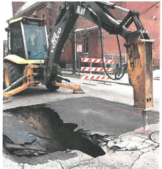
Crews work to repair a sewer collapse at Clay Street and Muhammad Ali Boulevard.
