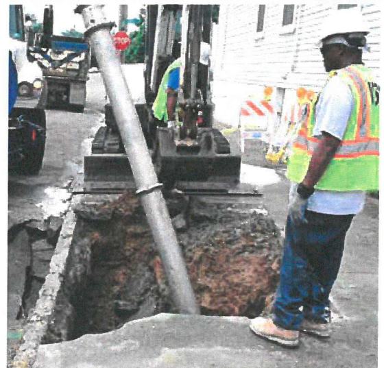
In May 2017, MSD Crews worked to clear debris from a cave-in on 25th Street.
