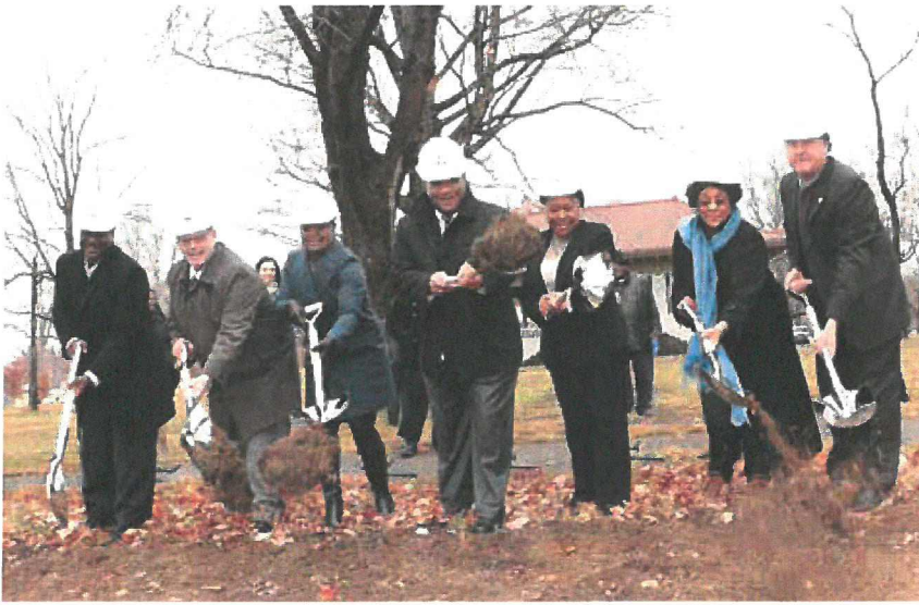
The dirt flies at the MSD Shawnee Park Basin Project groundbreaking event. Shown left to right: Eric Browne (Browne E&C Services), Matthew Ulliman (Ulliman Schutte Construction), Sadiqa Reynolds (Louisville Urban League), Tony Parrott (MSD Executive Director), Joyce Horton Mott (MSD Board), Cheri Bryant Hamilton (Louisville Metro Councilwoman, District 5) and Marty Storch (Metro Parks Deputy Director).
