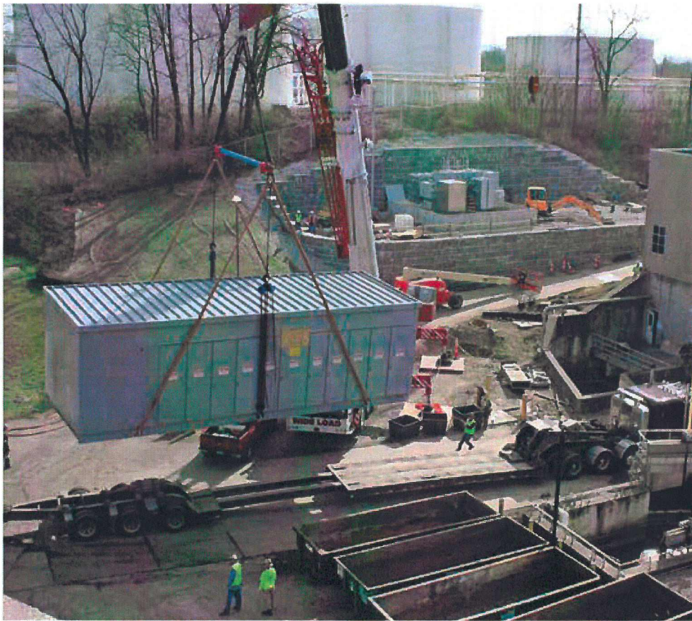
The new high-yard switch house is lifted from the transport truck bed.
