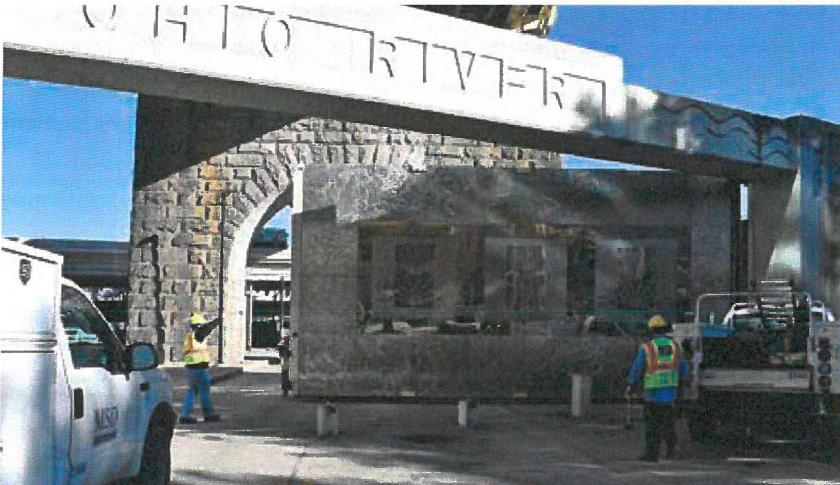
Above: MSD personnel practice closing the floodgate on Second Street near the KFC YUM! Center.
