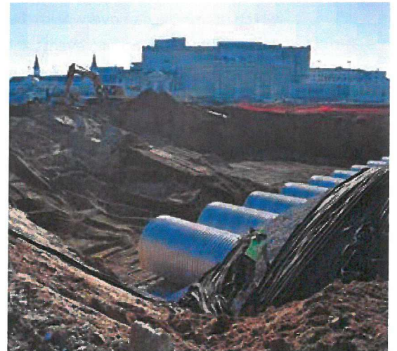
Above: Underground pipes at Churchill Downs will capture and infiltrate rainwater from the parking lot preventing this water from overwhelming the combined sewer system in this area. In a typical rainfall year, the pipes will capture 60 million gallons of rainwater.
