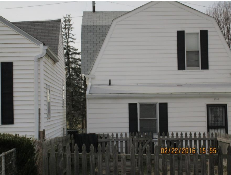
Looking due West at the rear of the home along the southern side of the property.
