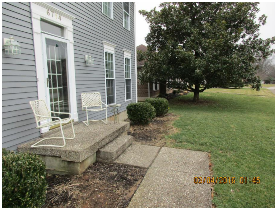
Looking Northeast at the front porch that would be built upon and out from the front of the home.
