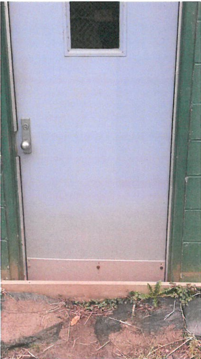
Maned Wolf Door—corrosion at bottom
