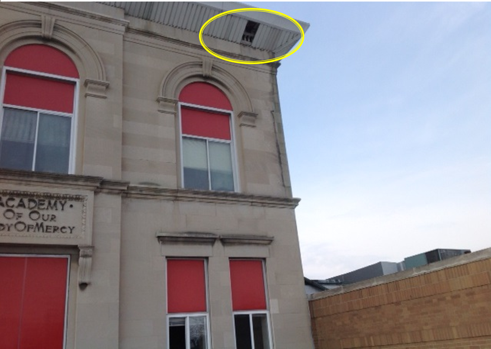
View of damaged soffit.
