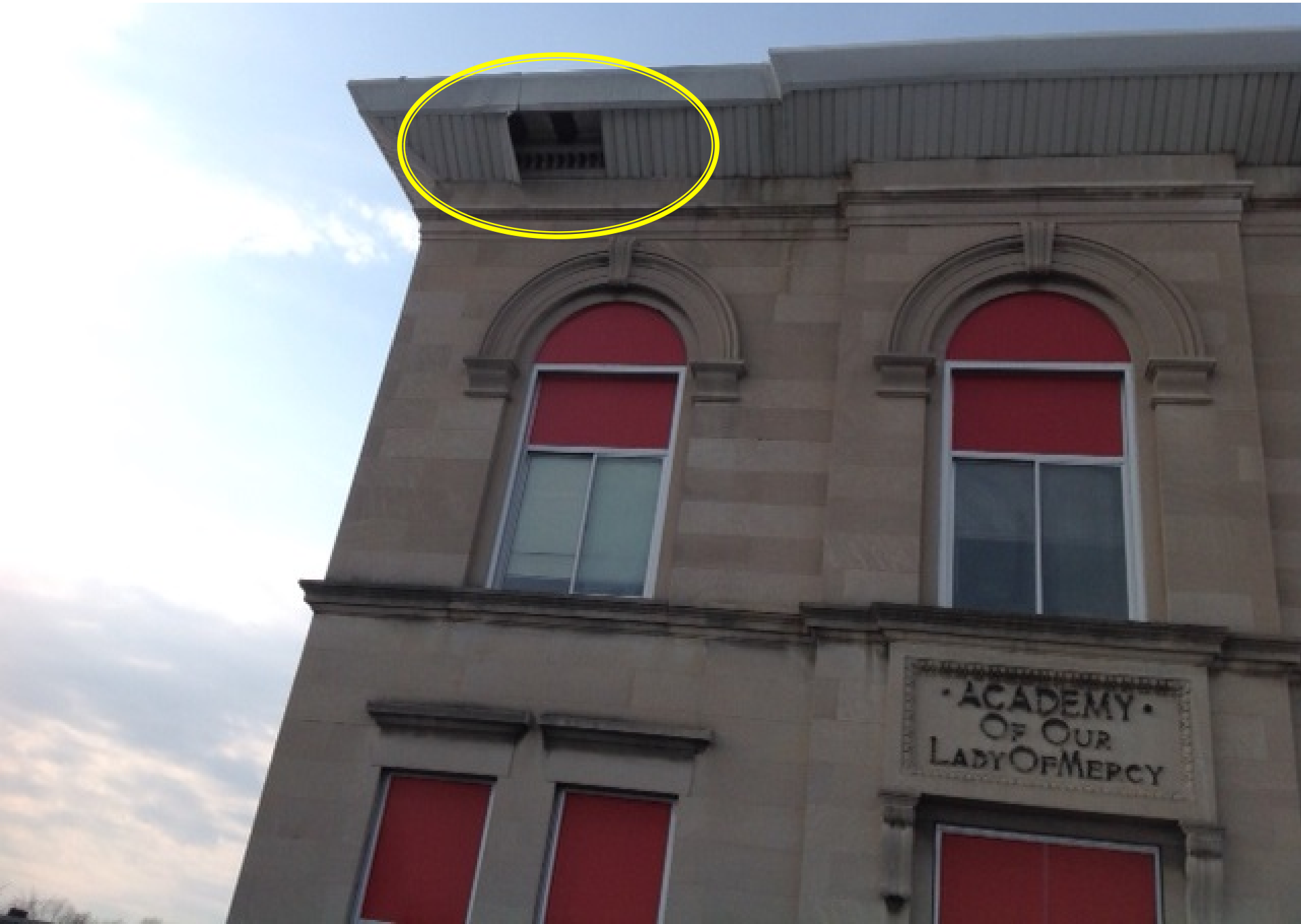
View of damaged soffit.
