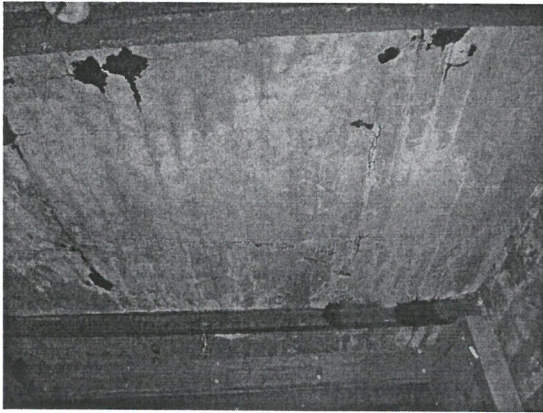
#5 spot breakage Not failed but close
