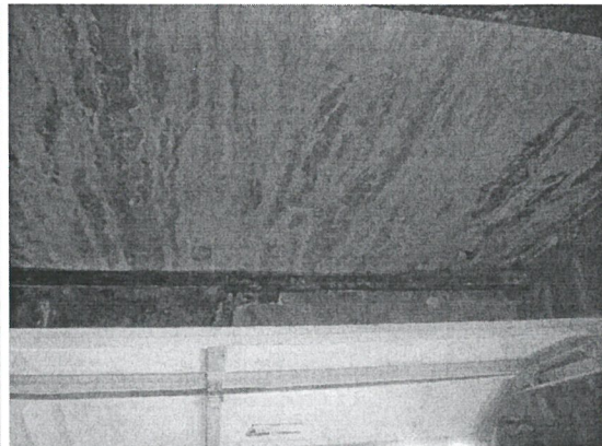
West side above door deteriorated
