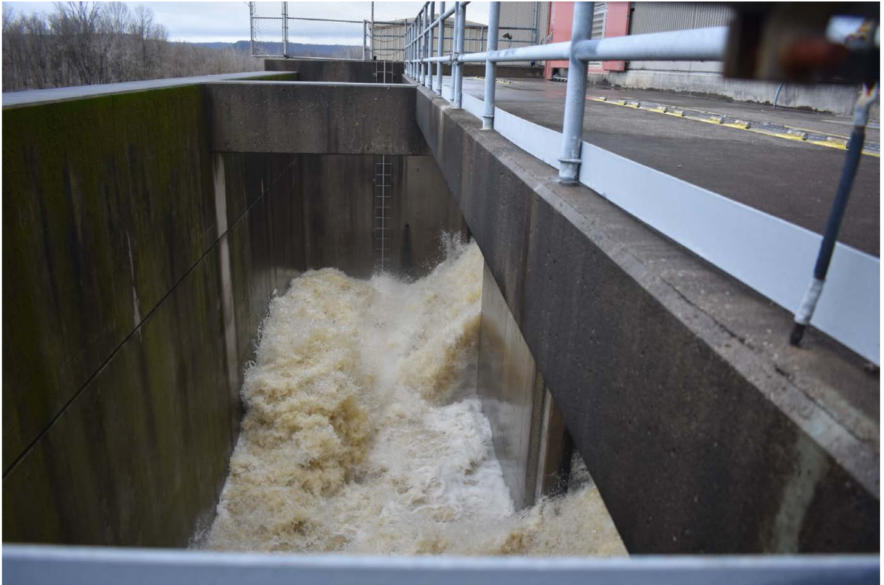
Pond Creek Flood Pump Station – 1.8 Million Gallons/minute
