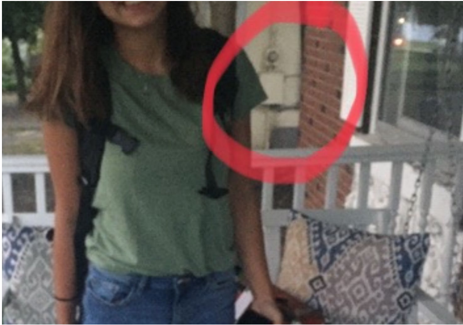
One electrical panel (photo dated August, 2018)
