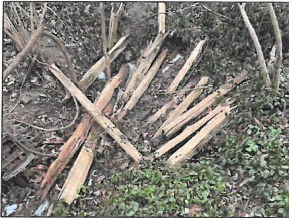
PHOTO NO. 9: Sinkhole at southwest corner (Feature 7)
