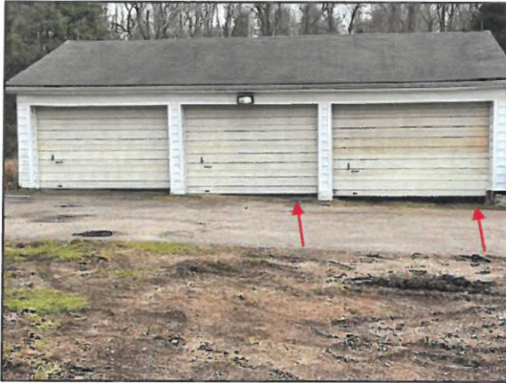
PHOTO NO. 11: Ground subsidence at garage
