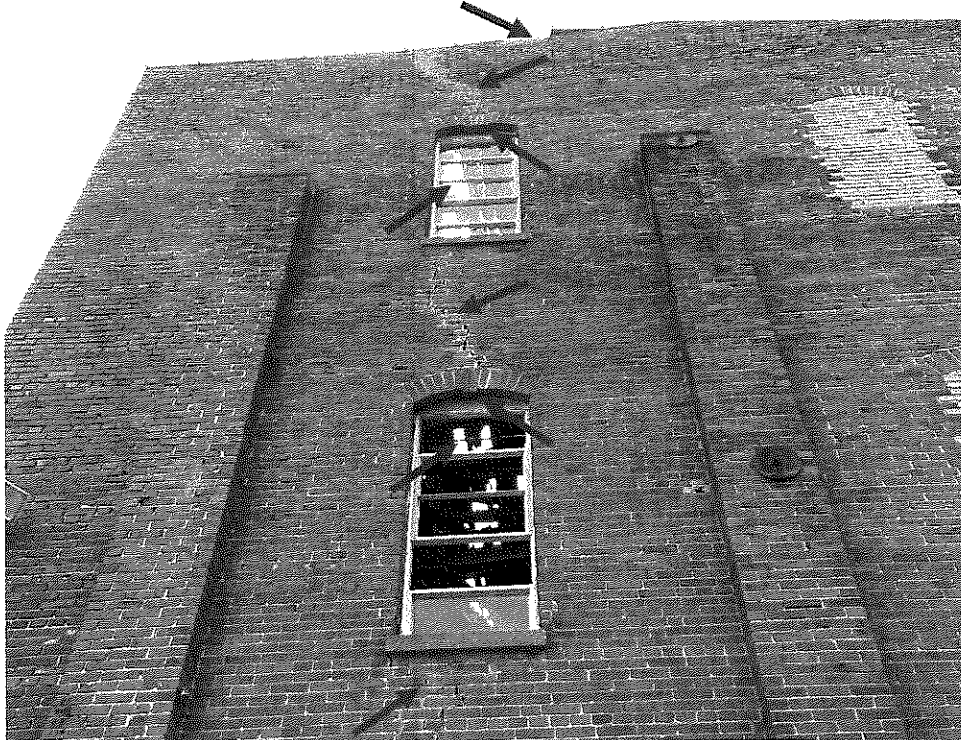
Photo 12 – West side of the northwest corner of the building. Missing cap at top of wall, cracks in old pointing repairs, and bricks in the arch tops of the windows about to fall. White spots seen in the windows are areas of collapsed roof.
