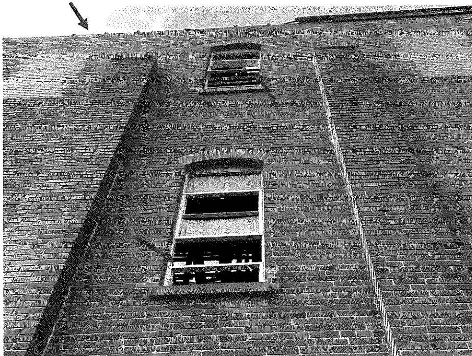
Photo 10 – North wall of the building. Missing gutters along most of the length of this wall due to deteriorated roof framing. Blue color in windows is collapsed sections of roof.
