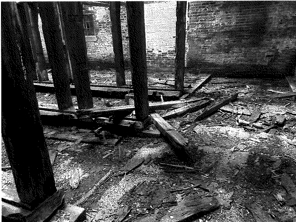
Photo 18 – More debris from collapsed roof. Most of the light in this area is from the collapsed roof.
