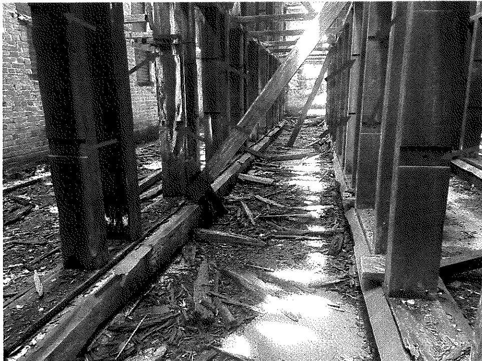
Photo 20 – Collapsed framing and debris from collapsed roof. Missing dunnage locations are easily visible. Third column on left has severe mold growth.
