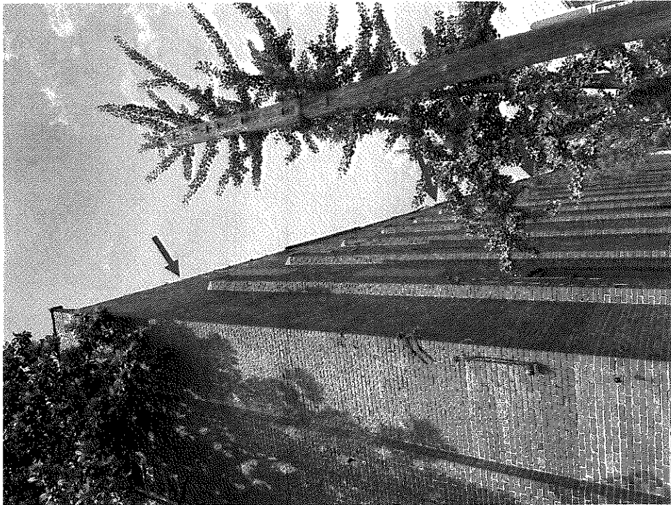
Photo 9 – Northeast corner of the building. Missing gutters along most of the length of this wall due to deteriorated roof framing.
