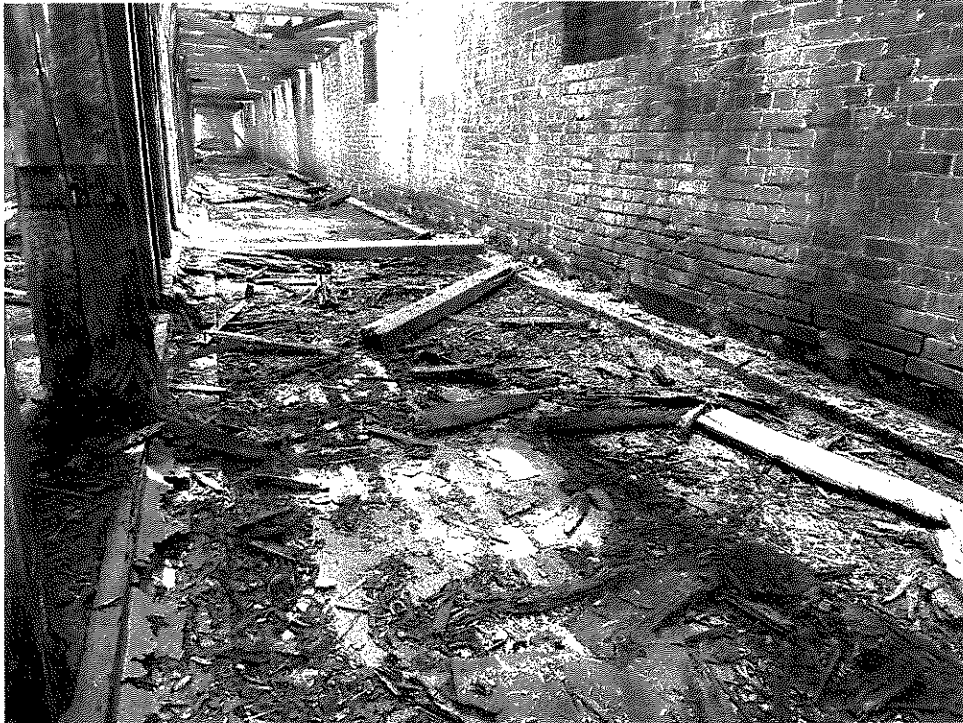
Photo 21 – Debris from collapsed framing on the floor and has broken a framing member at the next level up. Base of column is severely deteriorated.
