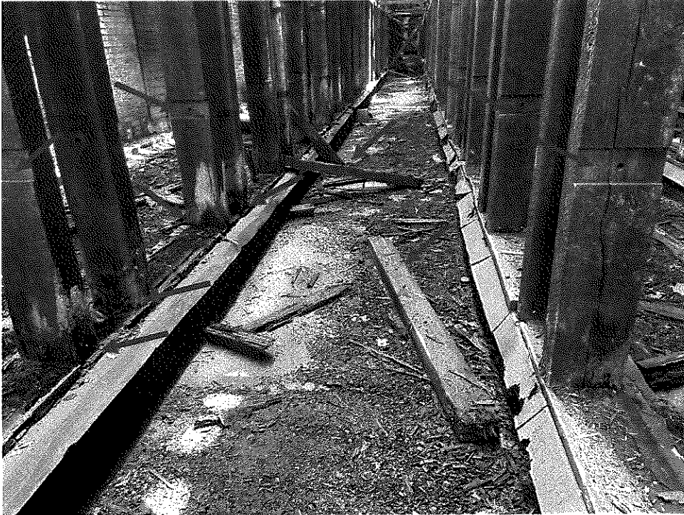
Photo 17 – Deteriorated post bases and debris from collapsed roof above. The notches in the posts with the hole in them are the locations where the 4x4 dunnage should be.
