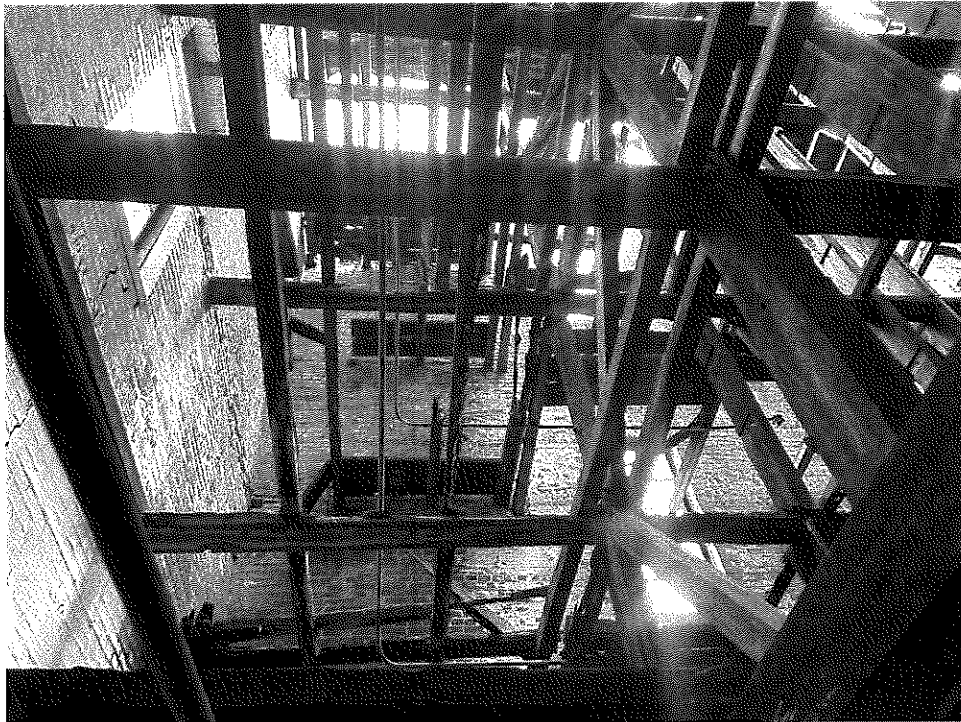
Photo 14 – Interior wood framing with deteriorated and molded wood. Large area of collapsed roof is visible.
