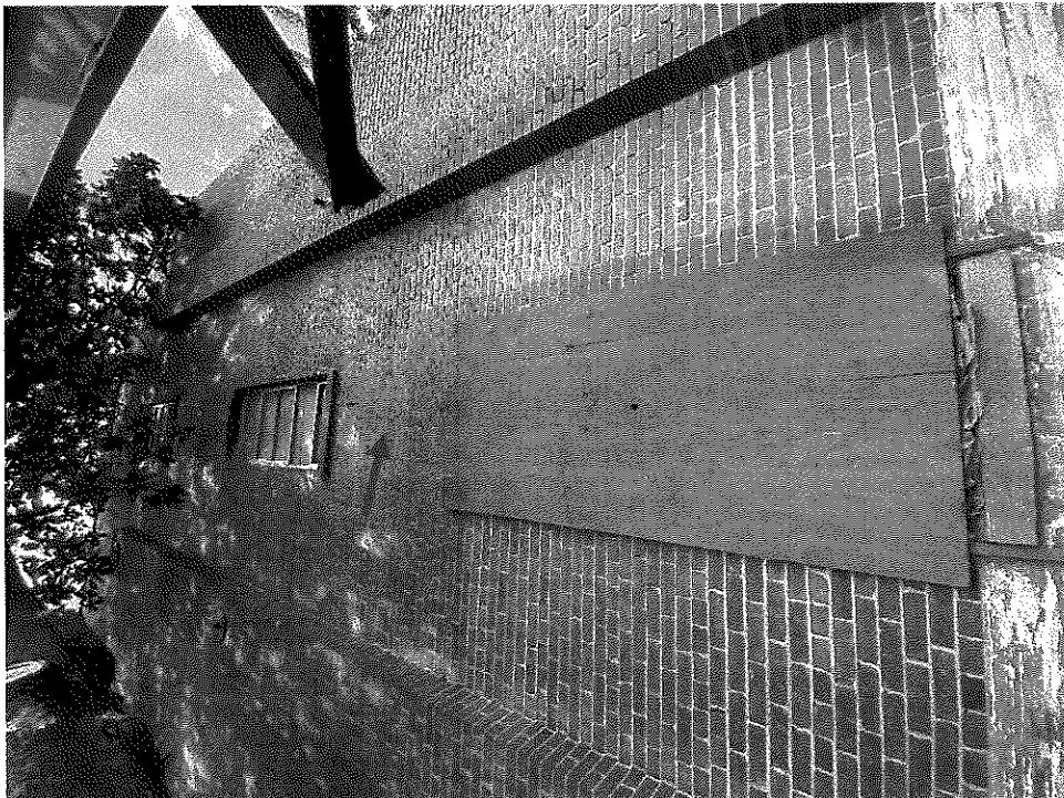
Photo 8 - East side of the northeast corner of the building. Cracks extending up the height of the wall and loose bricks over the lower arch top window.
