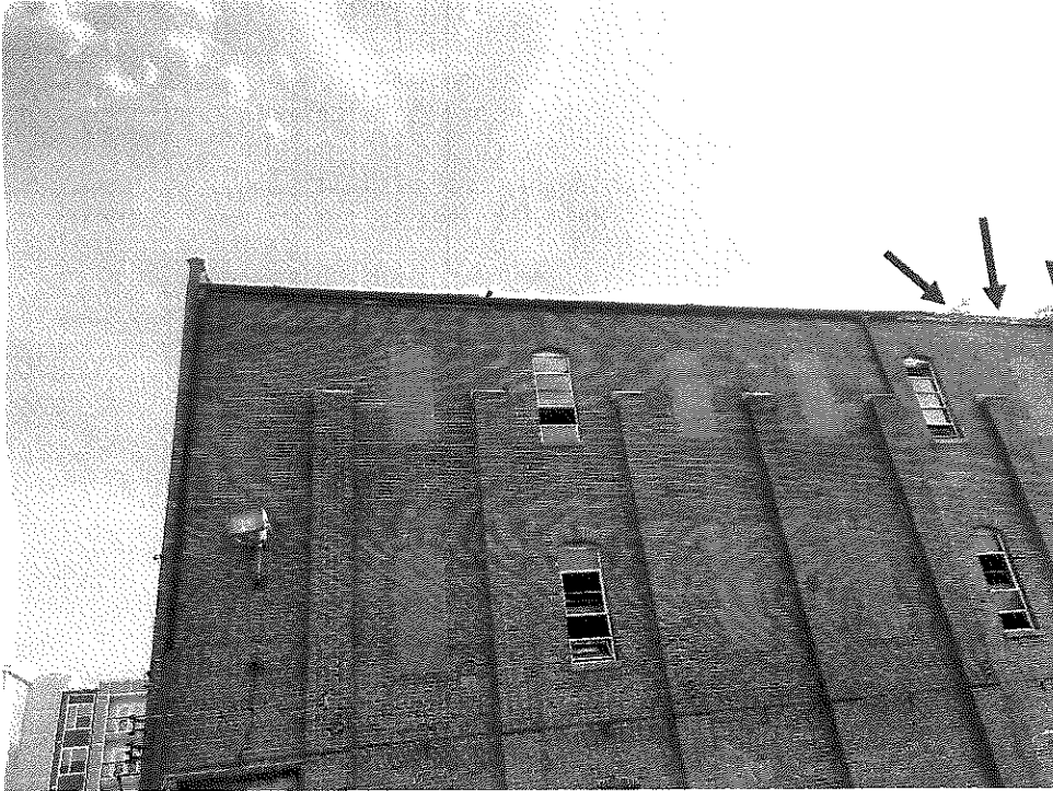
Photo 1 - South side of the southwest corner. Large plant growth is visible. Missing gutters from deteriorated roof framing.
