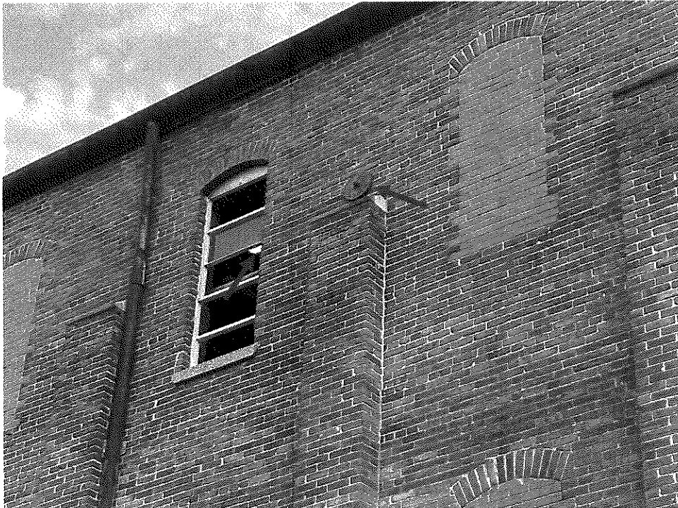
Photo 4 - South side of building. Tension cable plate is not flush to the face of the brick wall. White spot in window is the edge of an area of collapsed roof.
