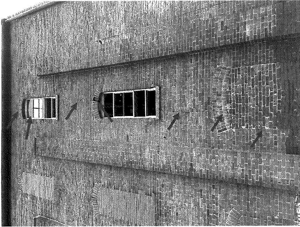
Photo 5 - South side of the southeast corner of the building. Past pointing work has cracked at top arch top window and cracking extends down wall. Dislodged brick in lower arch top window is about to fall. Blue in top window is collapsed roof.
