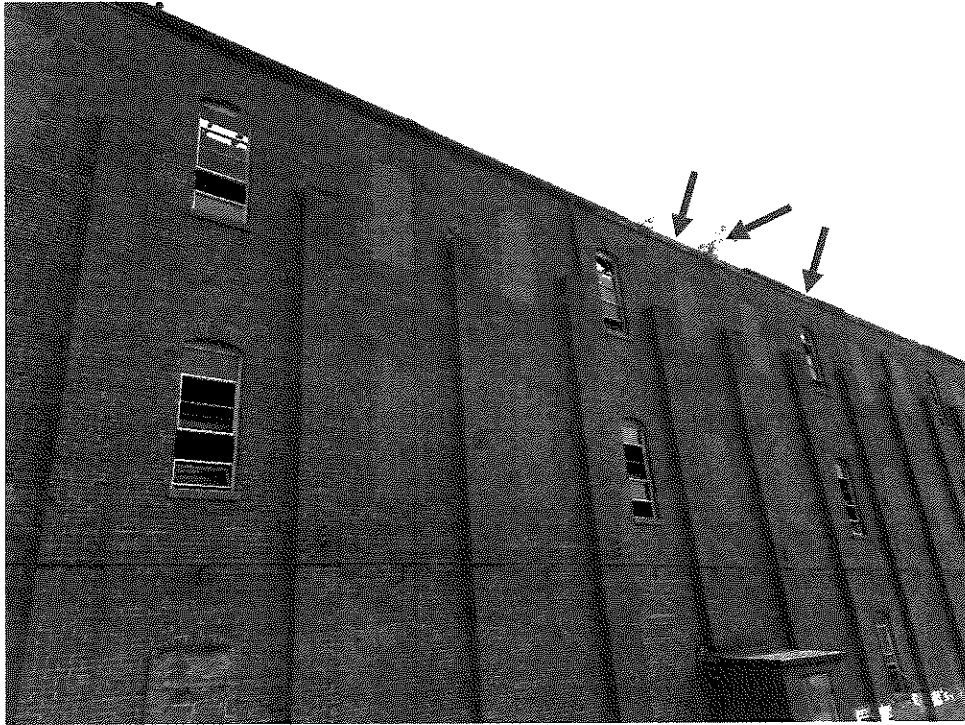
Photo 3 - South side of building. Large plant growth is visible. Missing gutters from deteriorated roof framing. White spots in upper windows are areas where the roof has collapsed.
