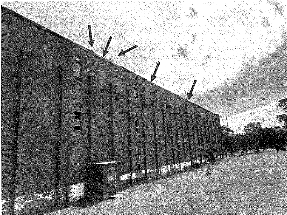
Photo 2 - South wall of the building. Large plant growth is visible. Missing gutters from deteriorated roof framing.
