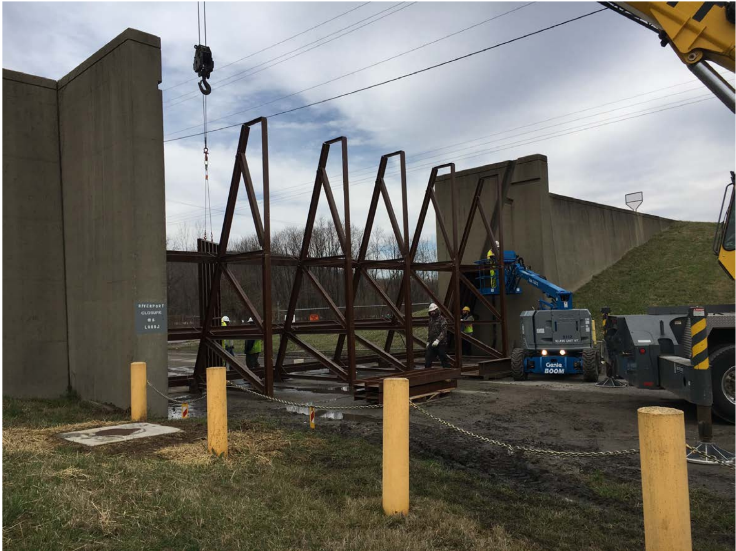
Port Road Floodwall Closure – Riverport
