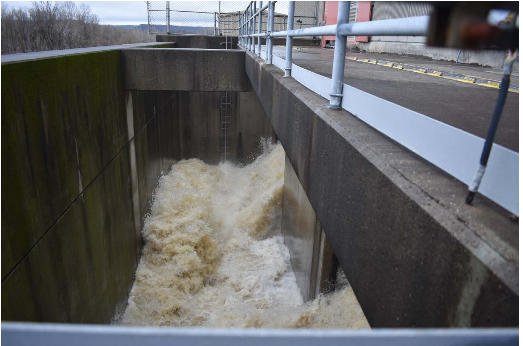
Pond Creek Flood Pump Station – 1.8 Million Gallons/minute
