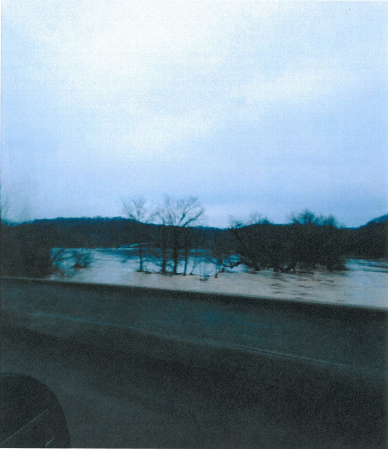
Bardstown Road Bridge with water dangerously close to the top of the bridge. In the back ground is the Floyds Fork park bridge.
