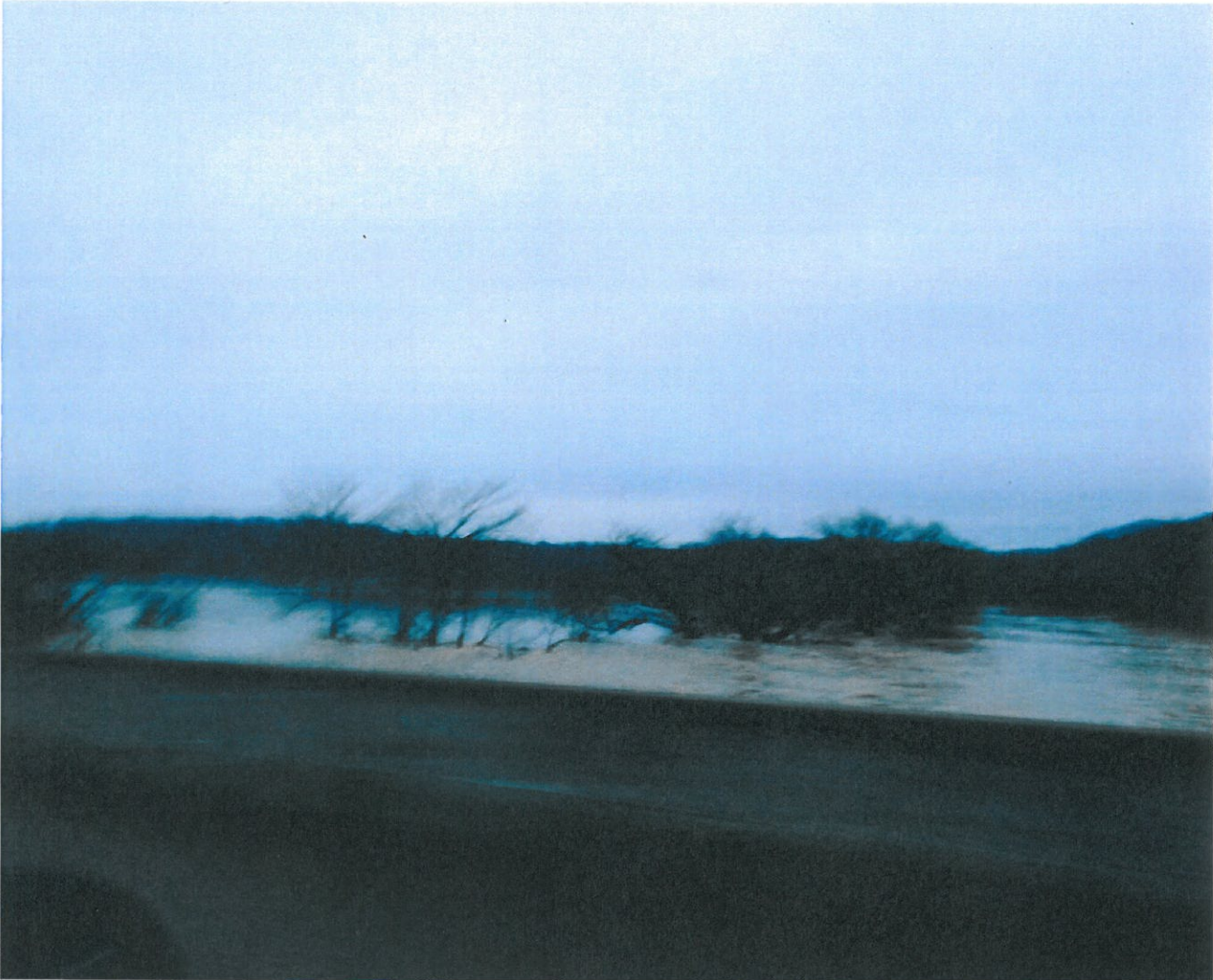
Bardstown Road Bridge – Water dangerously close to the bridge.
