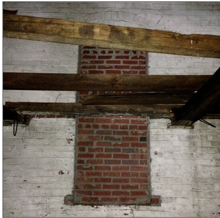
Bricked in Window Interior
