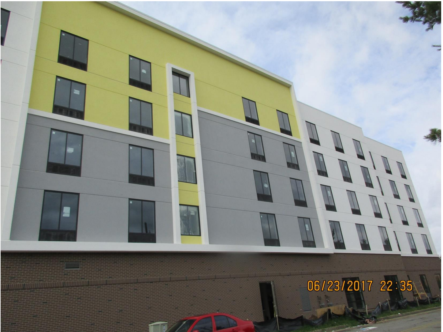
The location on the north façade where the signs are proposed to be installed.
