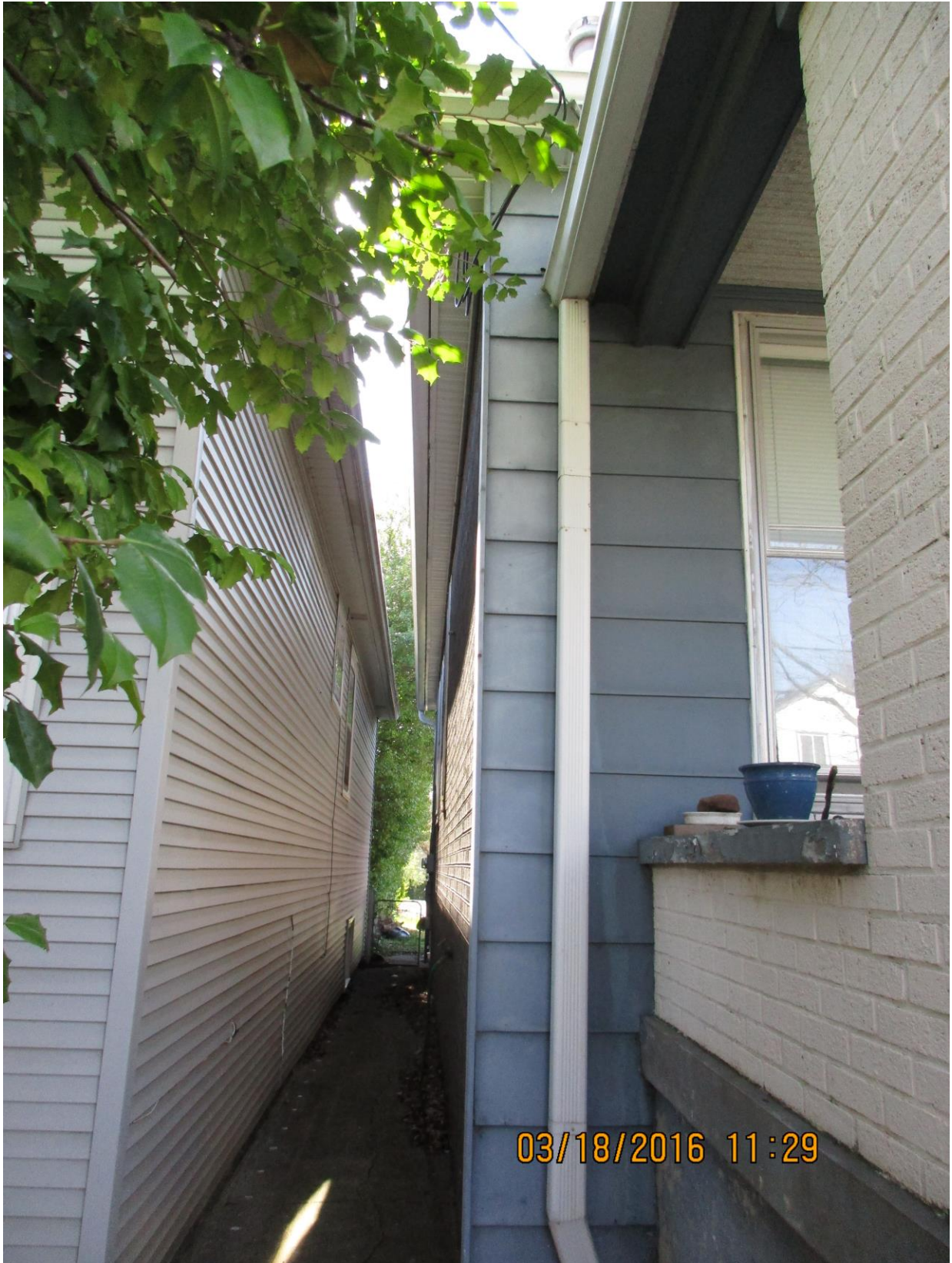
Looking down the walkway where the western property line between 1904 (left in photo) and 1902 (right in photo) Stevens Avenue. Notice the space between the gutters of each home.
