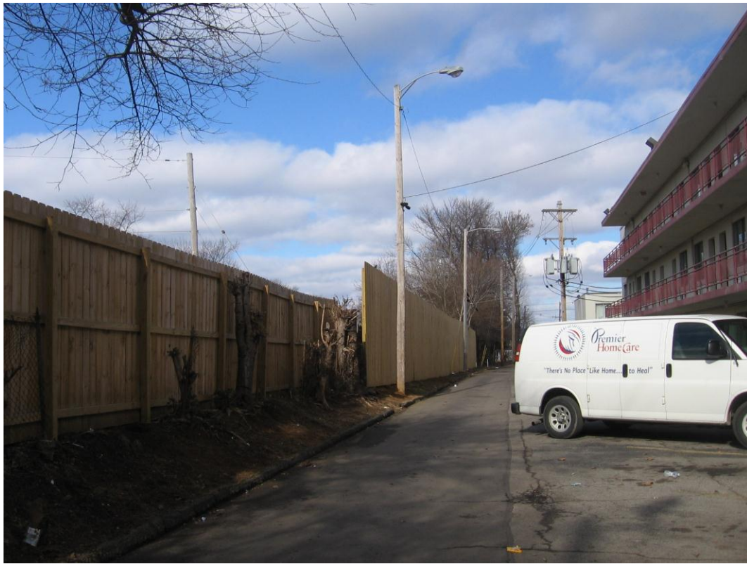
Southern Portion of the new fencing along the rear of the property
