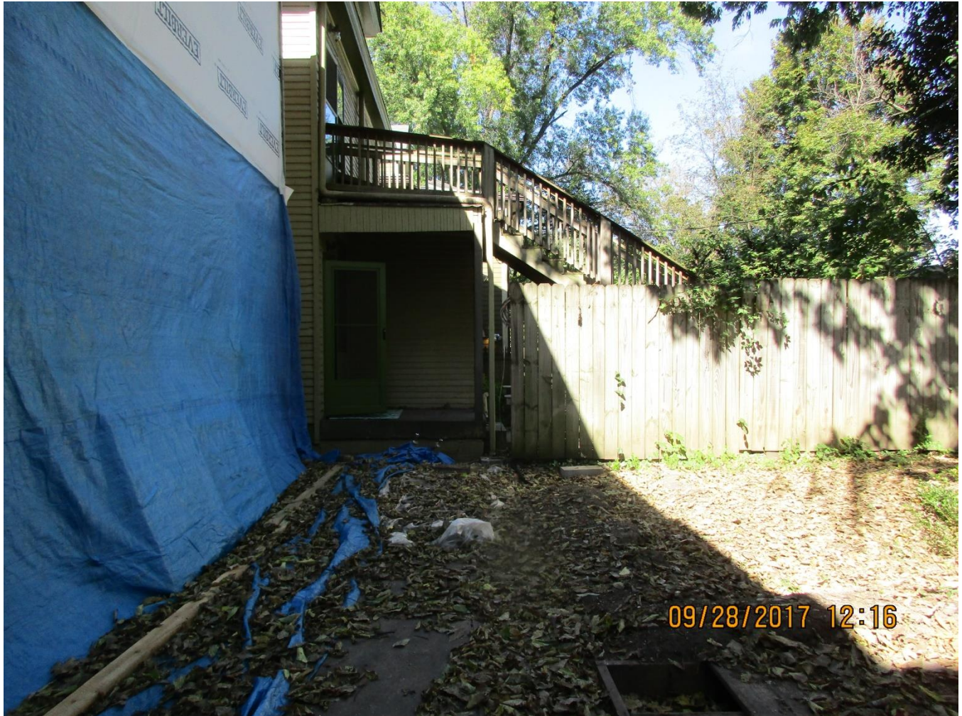
The rear of the principal structure where the addition is proposed to be constructed. The encroachment is proposed near the fence.
