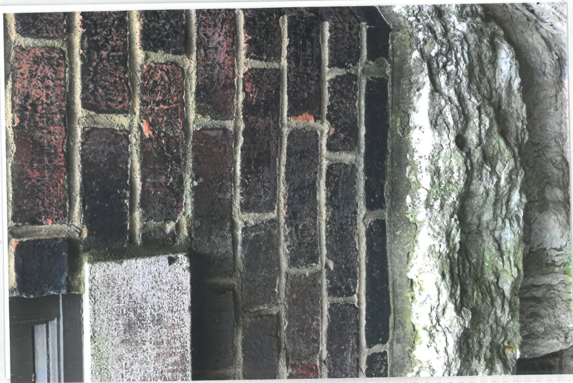
1214 S. Brook St window sill, brick, block
