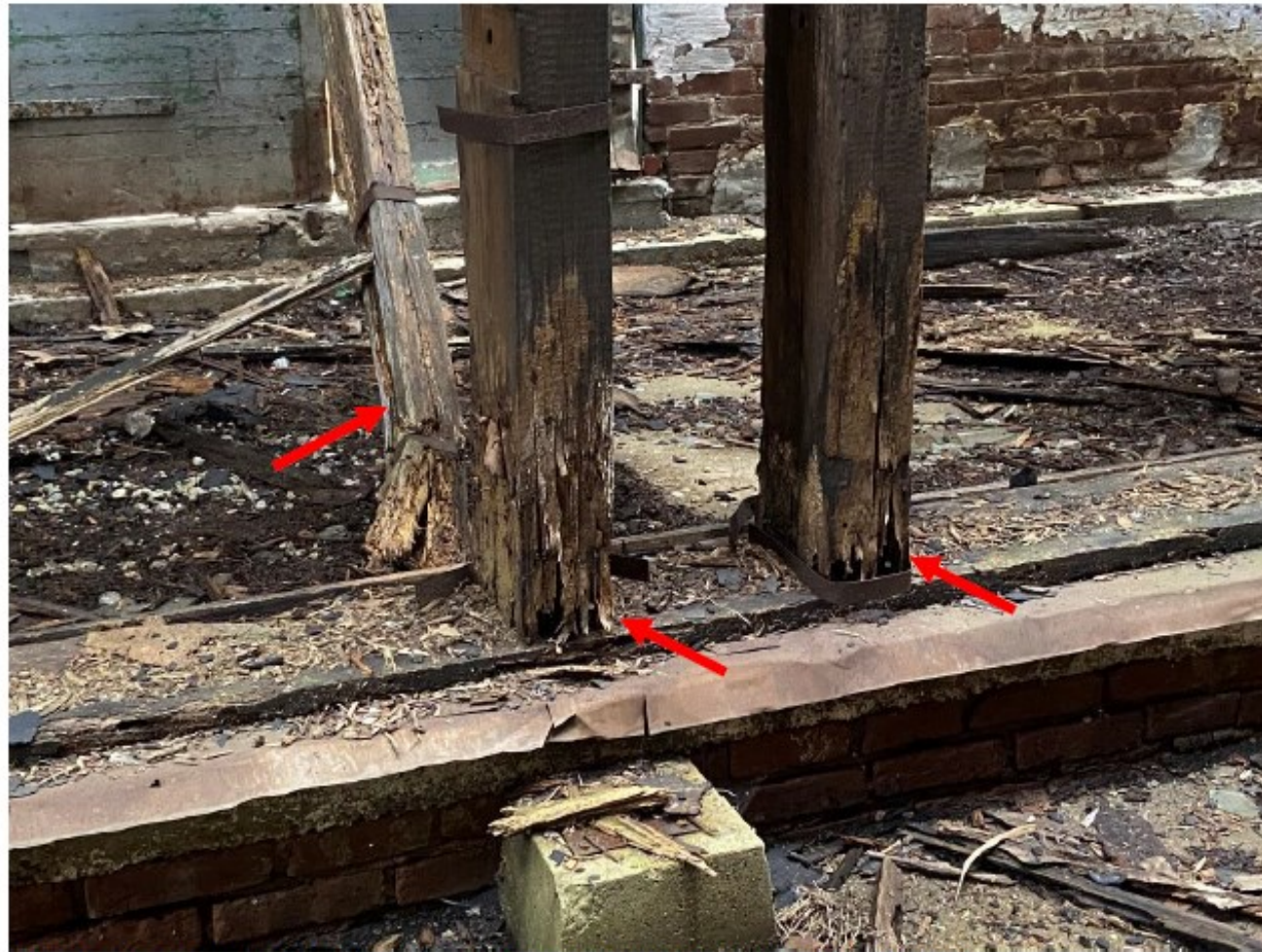
Photo 15 – Collapsed beam and severe deterioration at the base of two (2) posts.
