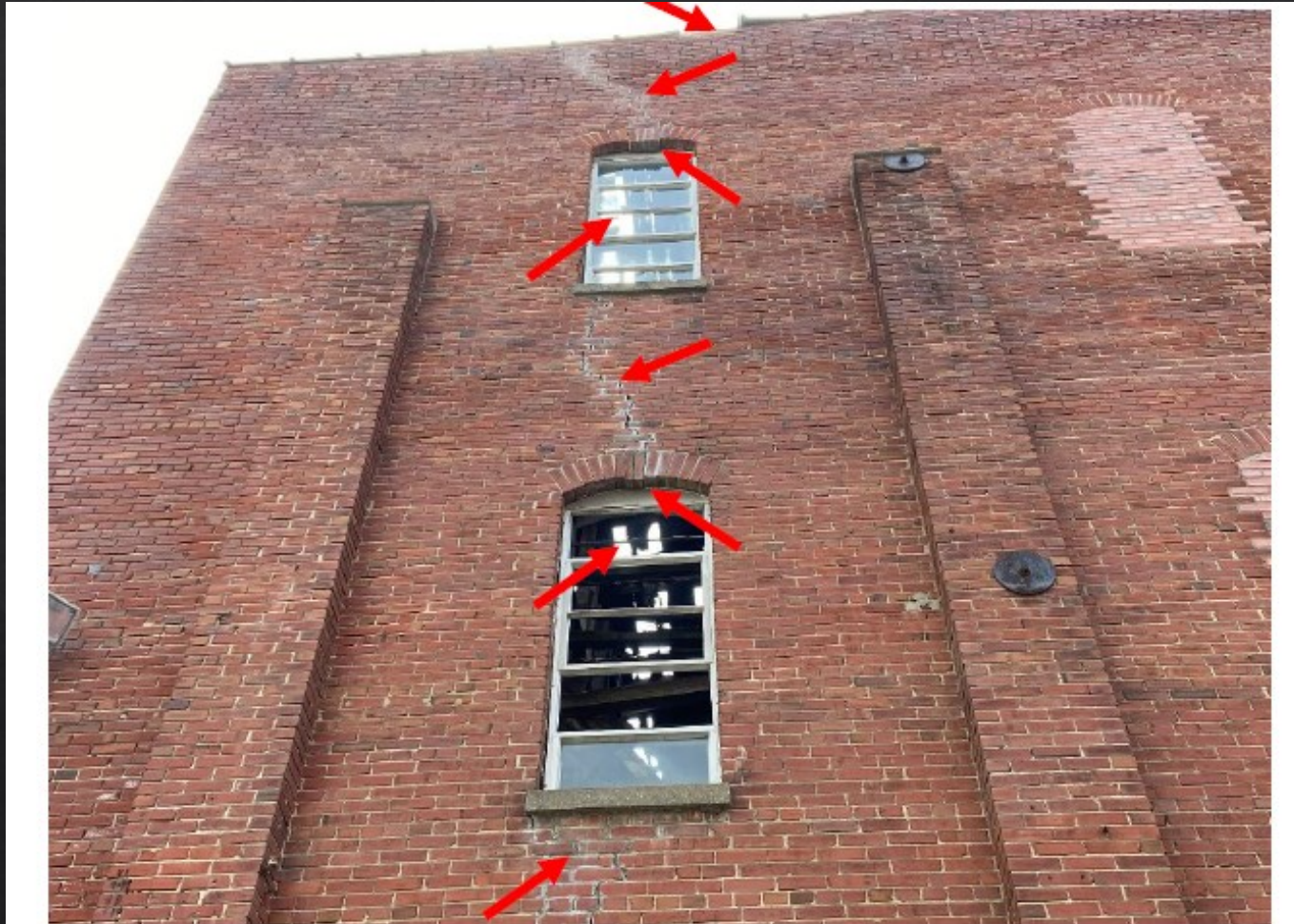
Photo 12 – West side of the northwest corner of the building. Missing cap at top of wall, cracks in old pointing repairs, and bricks in the arch tops of the windows about to fall. White spots seen in the windows are areas of collapsed roof.
