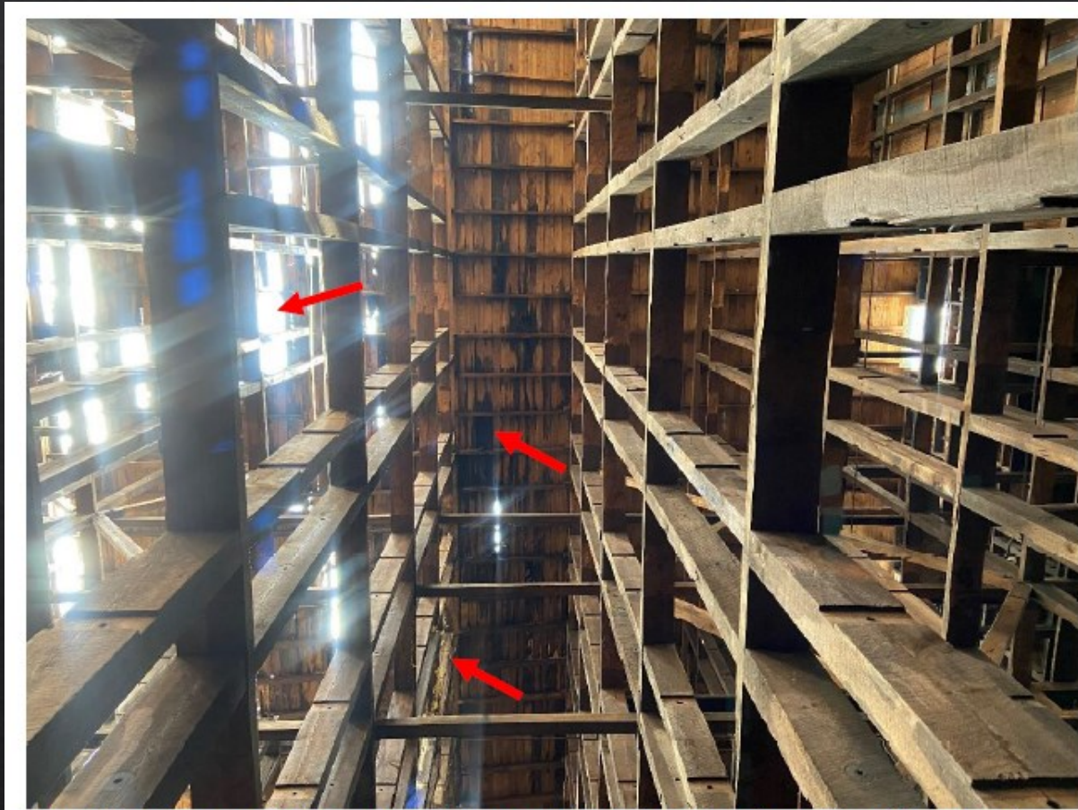
Photo 22 – Large area of collapsed roof. Deteriorated column in upper level of wood framing with severe mold growth. A better section of the visible roof with severe water damage. No 4x4 dunnage framing is visible; therefore, the posts are laterally unstable side-to-side.
