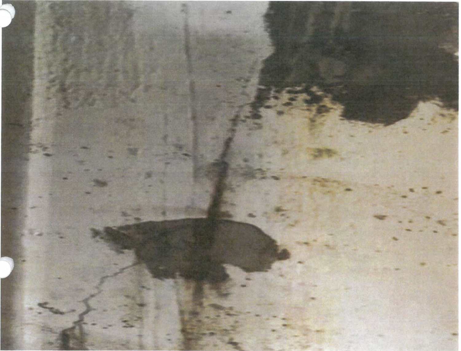
1999 - Cracked basement walls that were repaired by Mac Sawyers.
