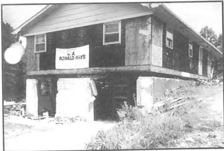
Jacking - preparing to move off basement 10" beam. Used Modern Hydraulics Power Pack & Black Jacks.
