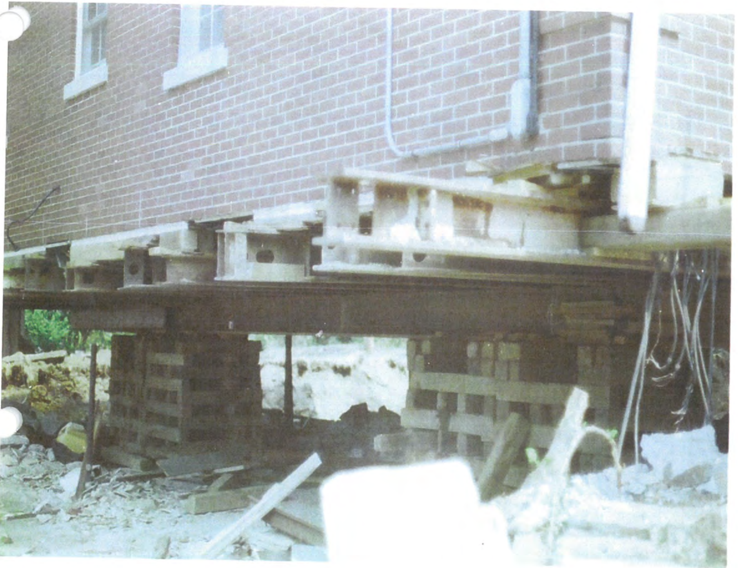
1992 - Mac Sawyers House and Building Movers job- House on cribbing being raised.
