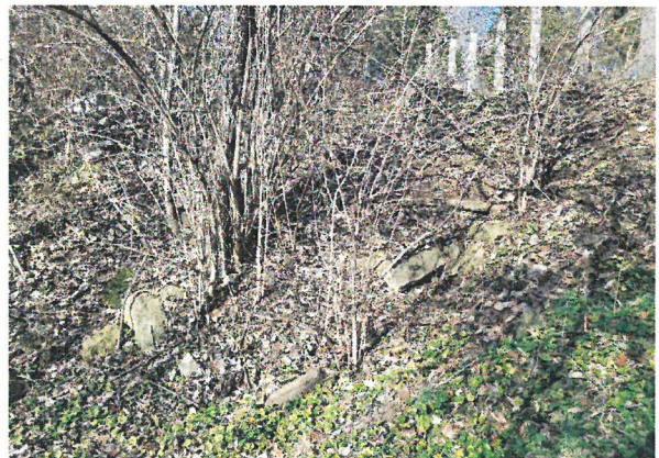
Area 01a – minor erosion
