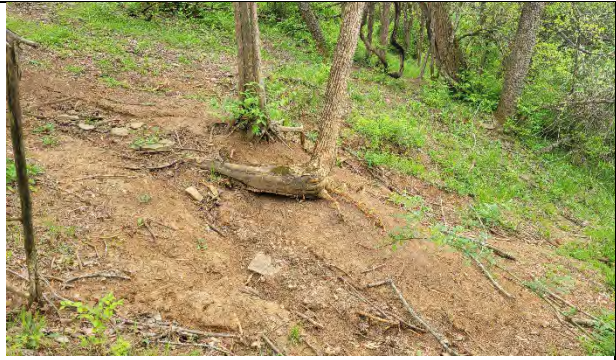
Photo 24: View of soil mounding, displaced cobbles, and minor erosion (Slope Area 10).
