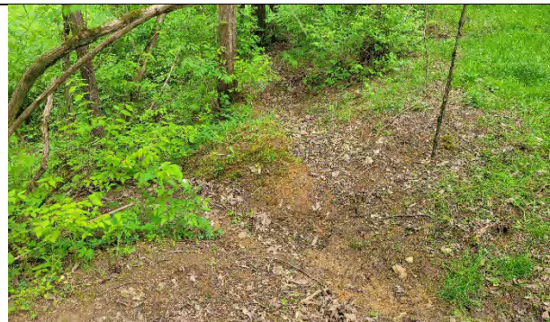
Photo 11: View of soil mounding, displaced cobbles, and minor erosion (Slope Area 7).
