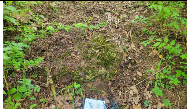
Photo 13: View of displaced cobbles (Slope Area 7).
