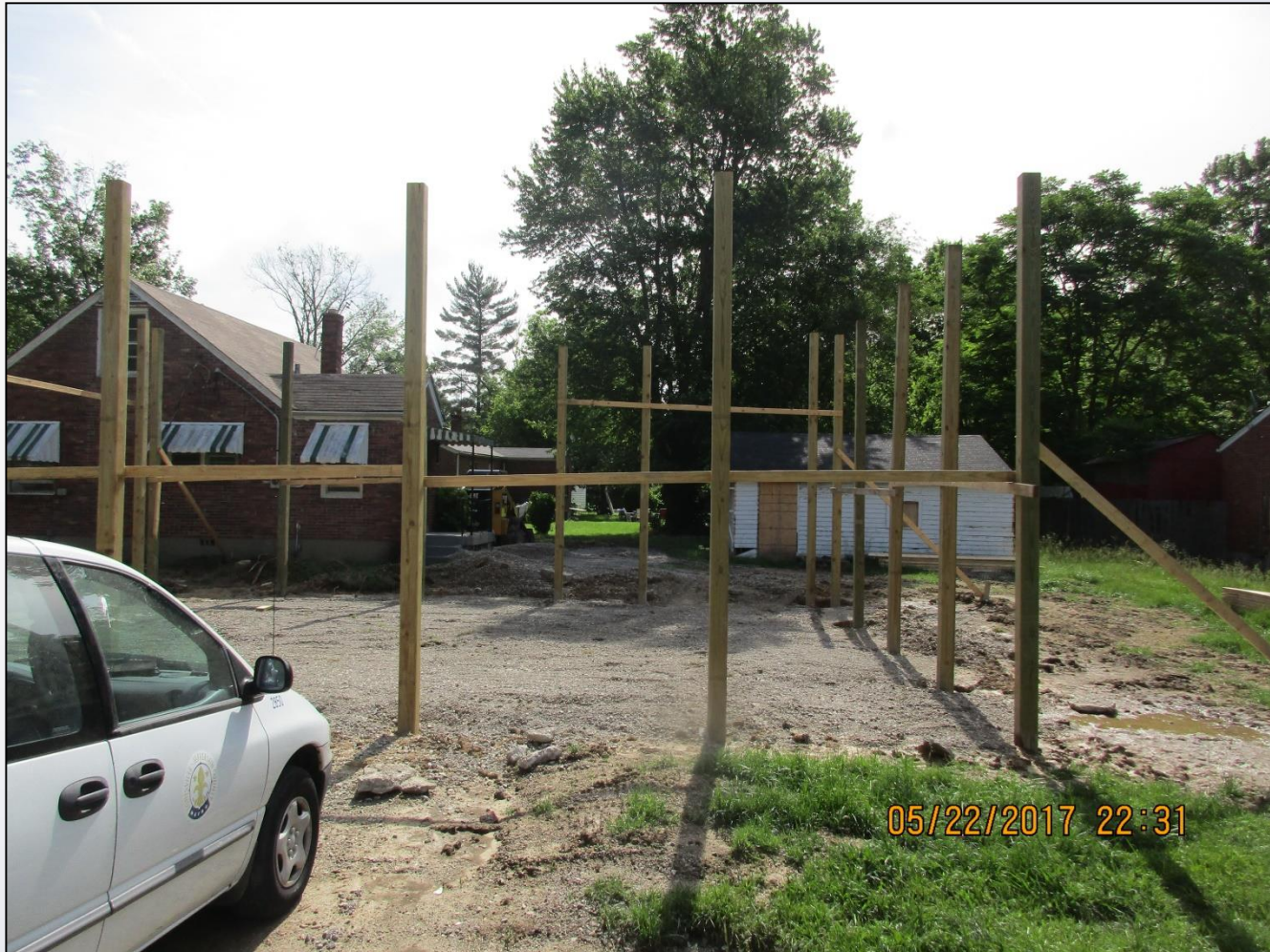
The partially framed pole barn and existing garage (garage to be removed)
