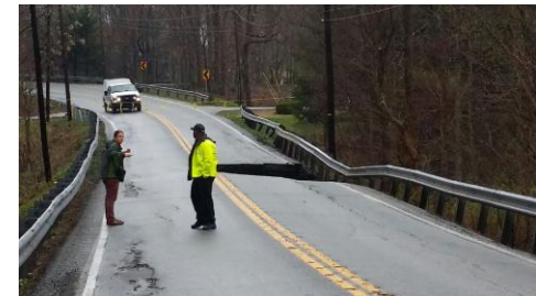
Road Washout on Hwy 22
