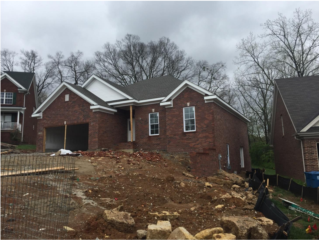
The side of the house where the encroachment occurs.
