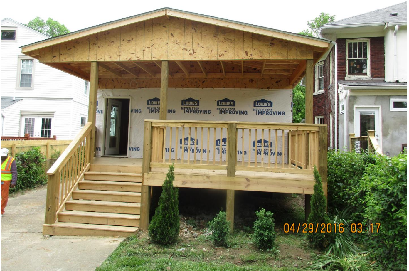
The rear addition (covered deck) that was issued a stop work order.
