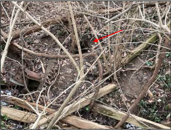
PHOTO NO. 10: Conduit/ swallow hole at Feature 7
