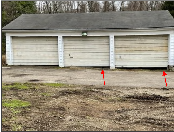
PHOTO NO. 11: Ground subsidence at garage
