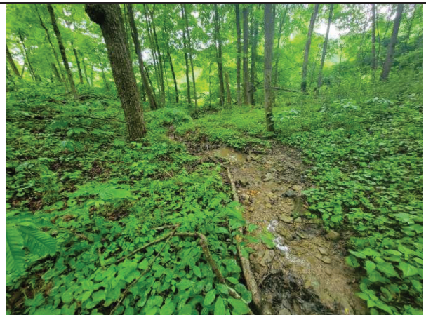
Photo 20: Additional drainage swale with displaced cobbles and slope profile (AOI-4).
