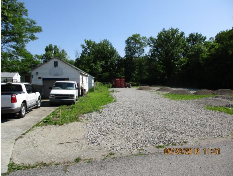
Looking along the western property where a 6 foot continuous screen would be required. Applicant is requesting a waiver (variance and waiver #5).
