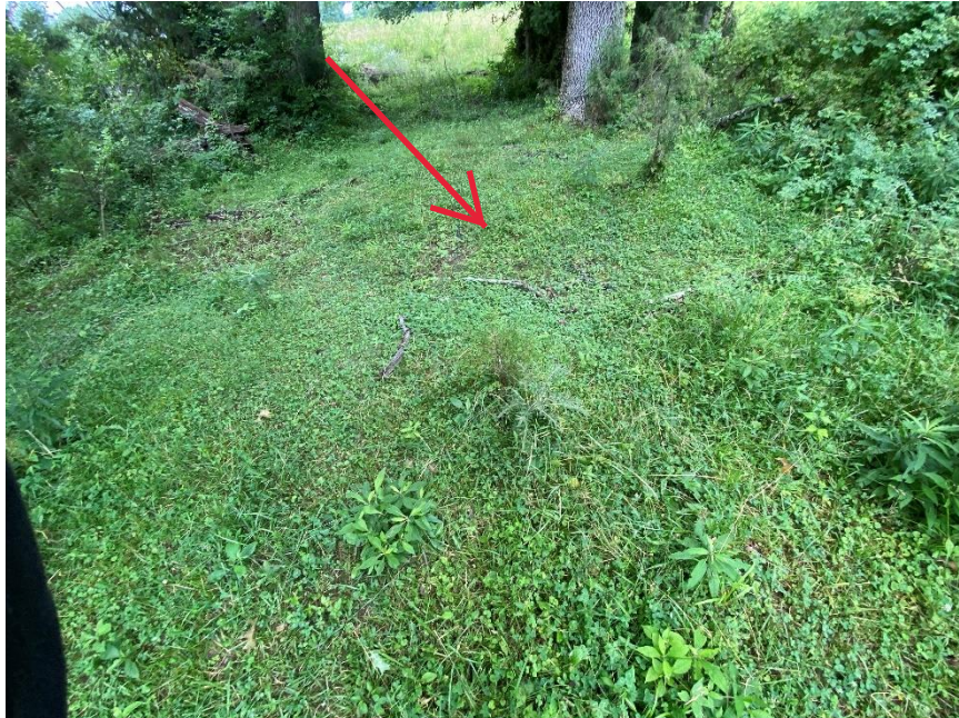
View of possible sinkhole shown as 4'x4'x1' depression (N 38.108780° W 085.684740°)
