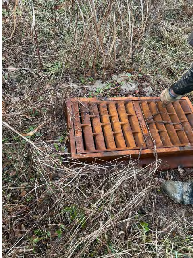
North Central Storm Sewer
