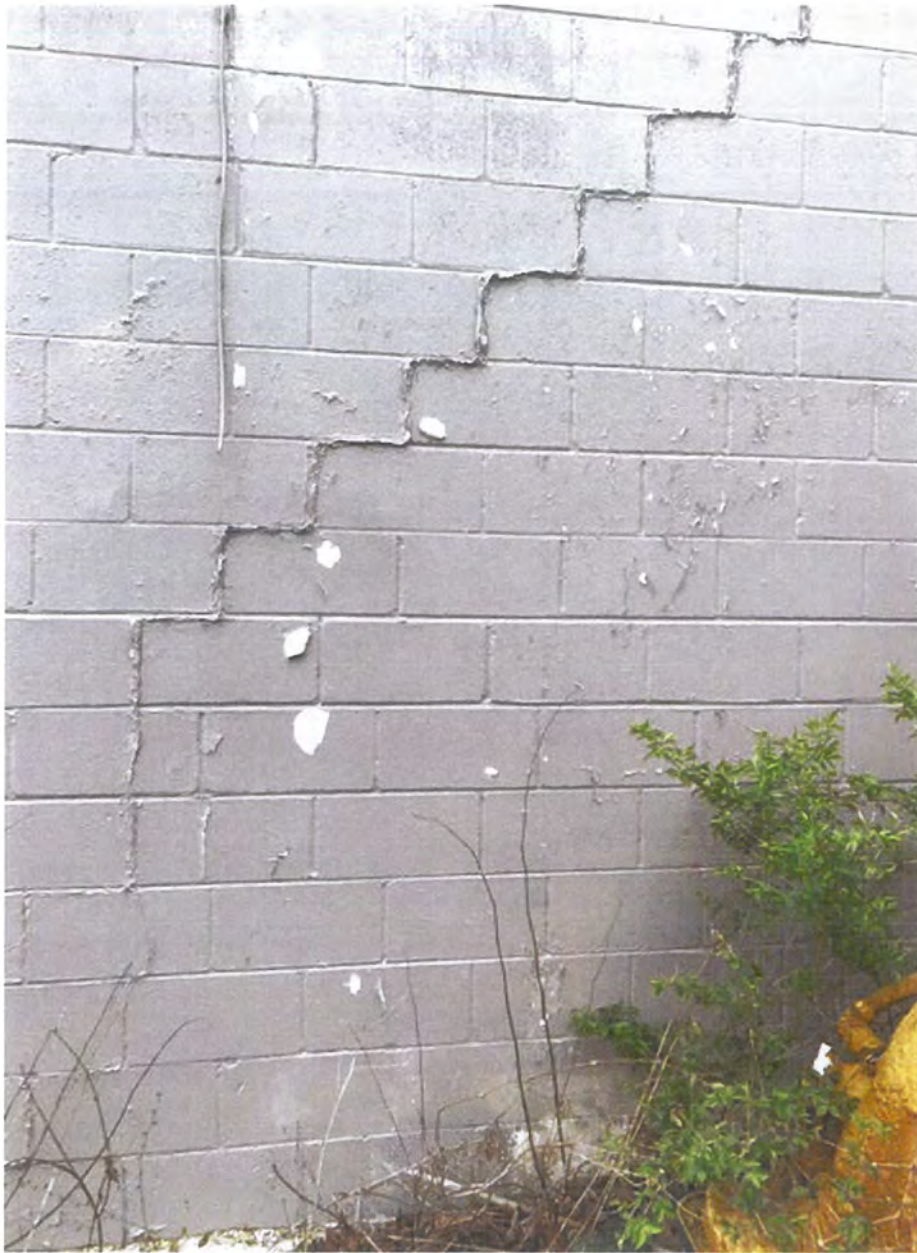
2007 - Failed foundation and masonry block repair on commercial building.
