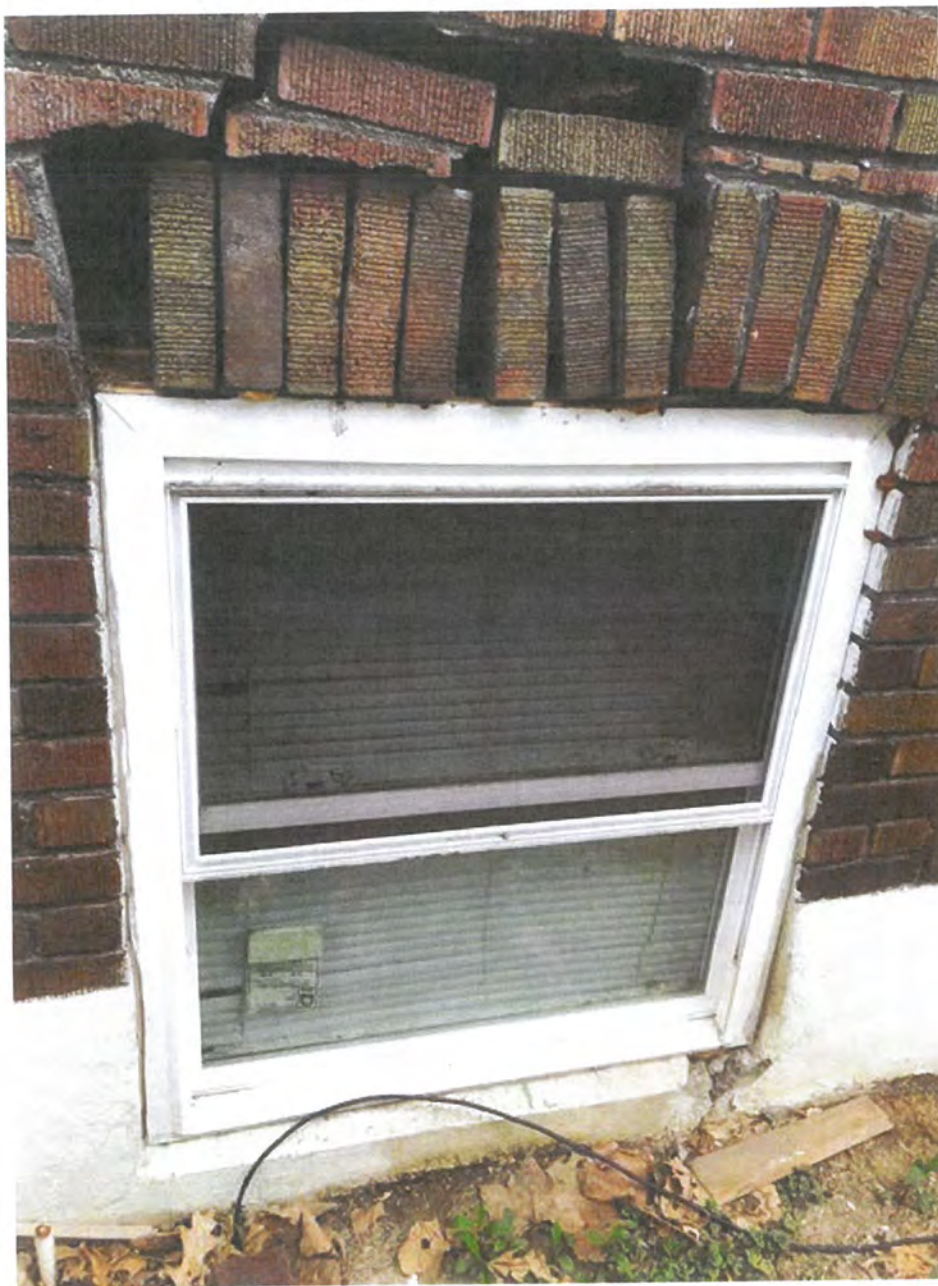
2012 - Foundation and brick failed.
