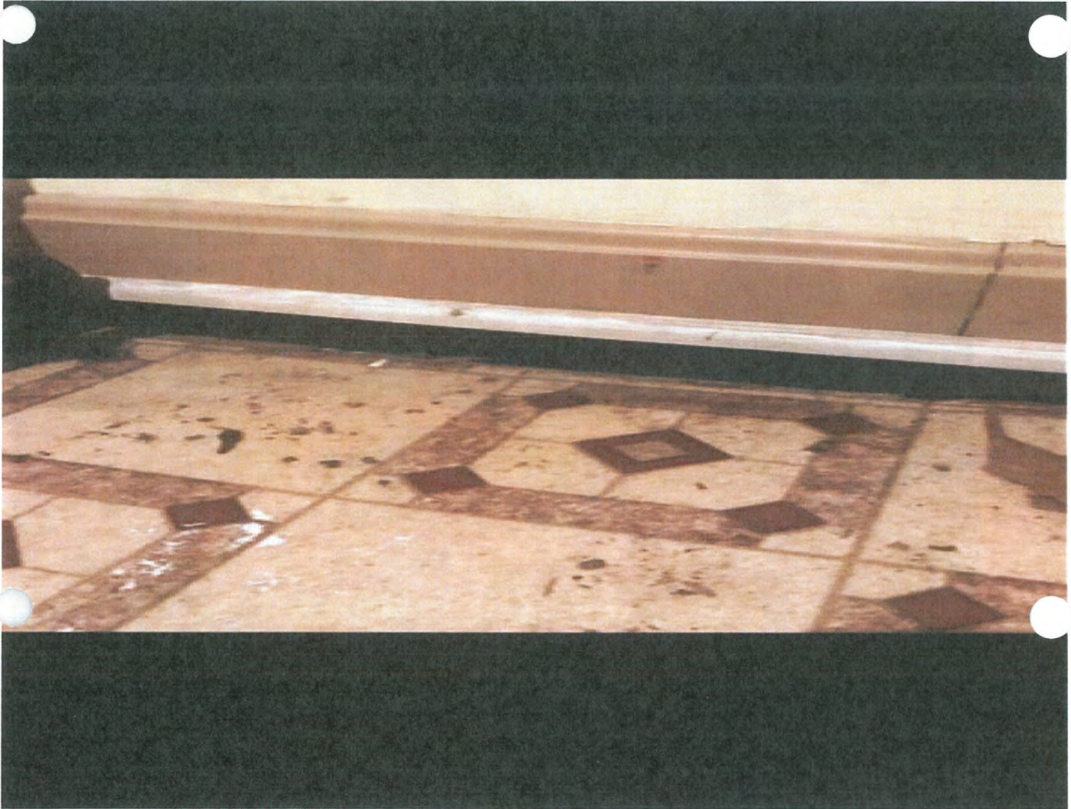
2009 - Unlevel floor prior to pier replacement.
