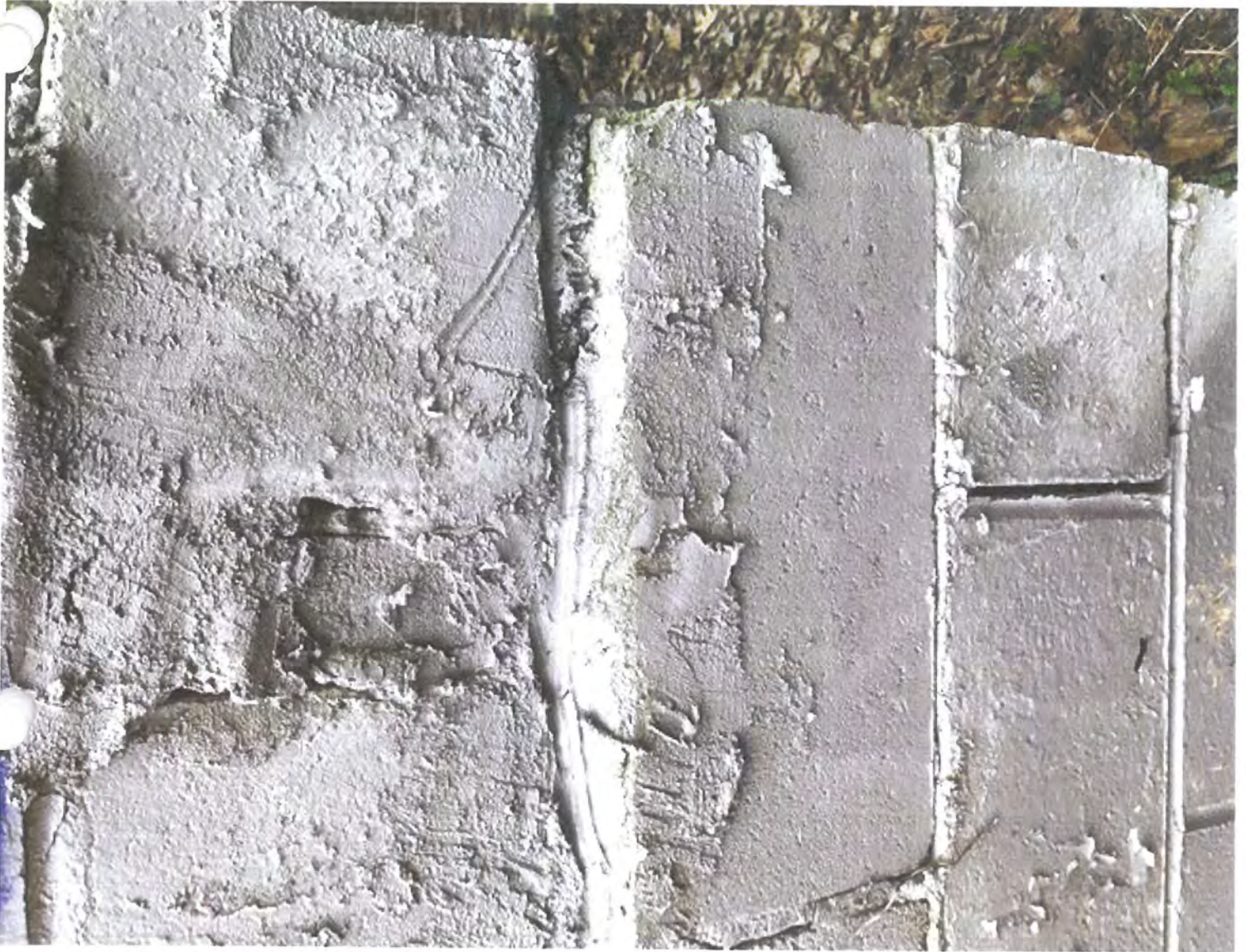
2007 - Failed foundation and masonry block repair on commercial building.
