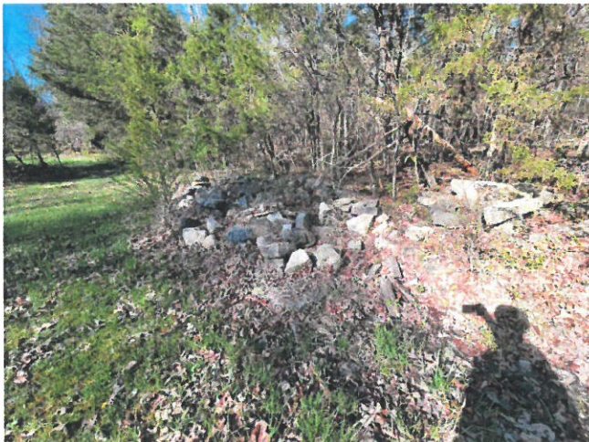
Photo 59 – View of typical rubble pile
