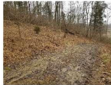
Access road and erosion at Lot 54
