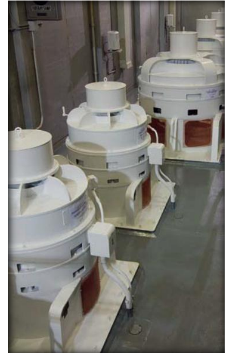
Pumps used to protect against Ohio River flooding.
