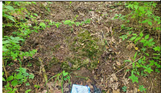
Photo 13: View of displaced cobbles (Slope Area 7).
