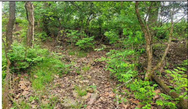
Photo 26: View of minor erosion, mounding, and "wedge shaped" slope failure (Slope Area 10).
