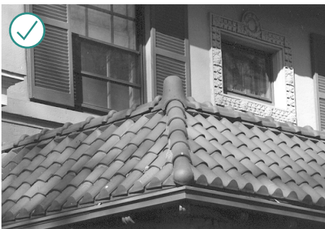
Use a replacement material that matches the color, texture, and character of the original roof material, and that has a similar proportion of seams and trim to the original roof material. When replacing a tile roof, try to reuse salvageable tiles on secondary roofs like porch roofs.
