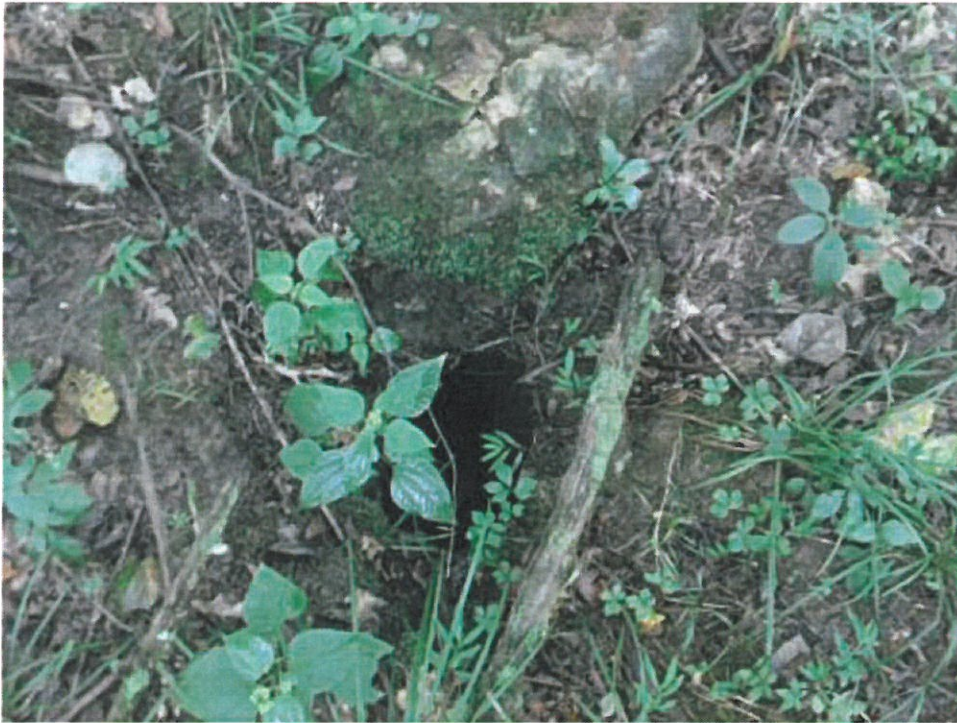
Potential Sinkhole Throat
