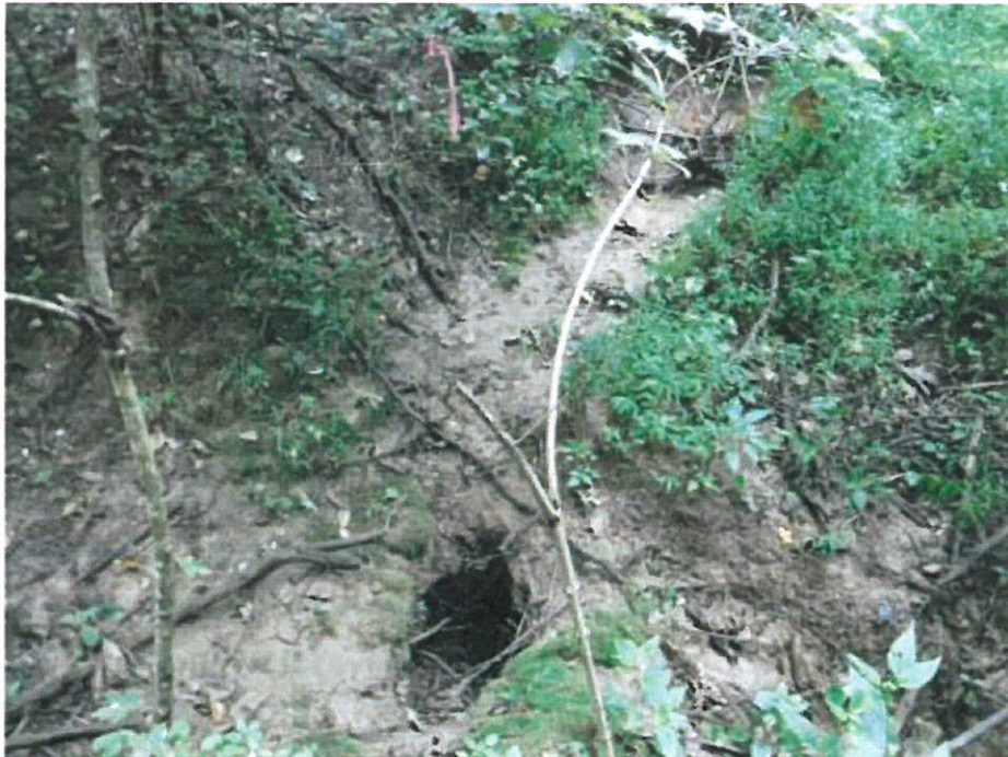
Potential Sinkhole Throat
