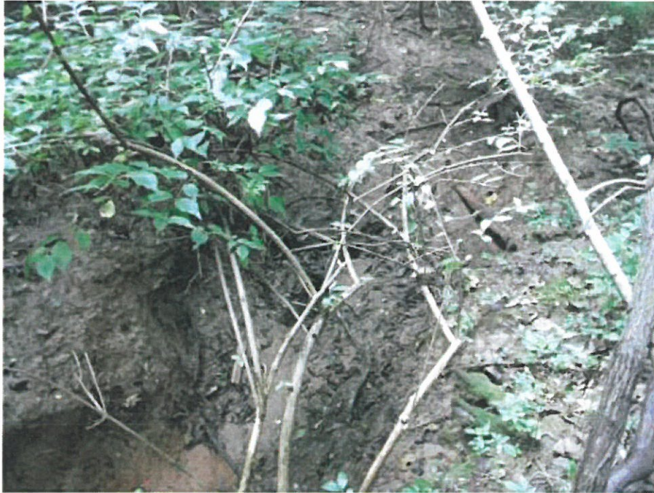
Potential Sinkhole Throat
