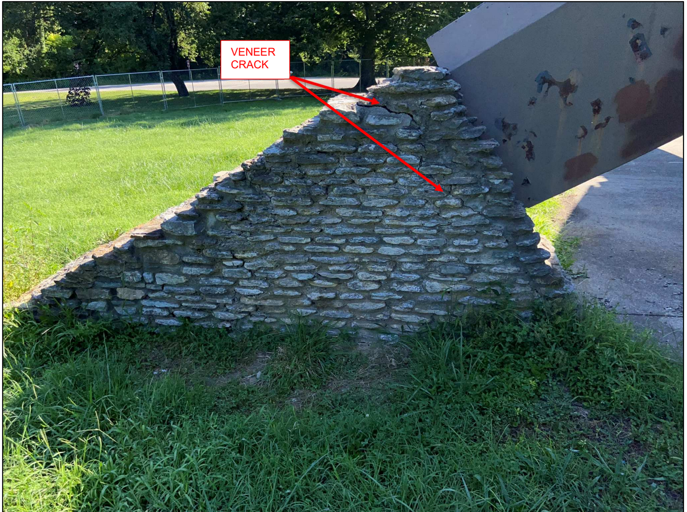
Photo 2: Abutment #8 Veneer Cracks
