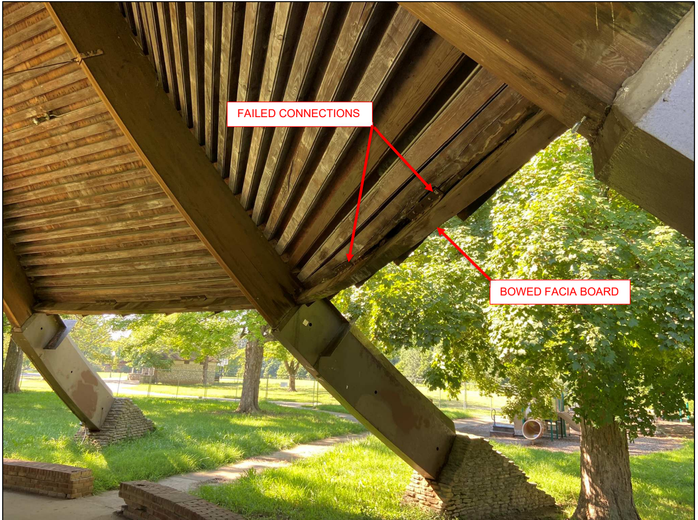
Photo 7: Bowed Fascia Board
