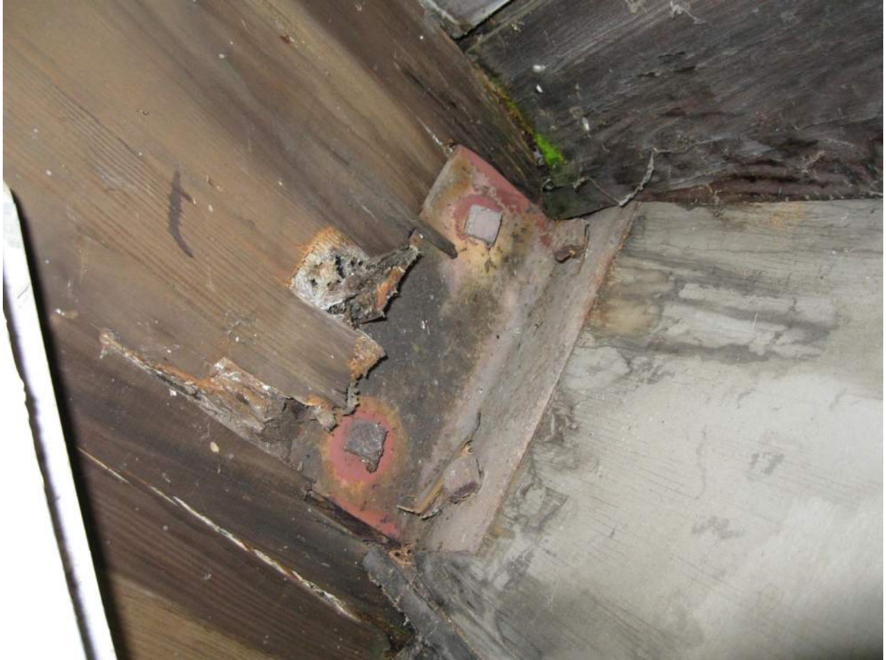
Photo 2 – Glulam arch wood decay near the connection of the horizontal roof framing members.
