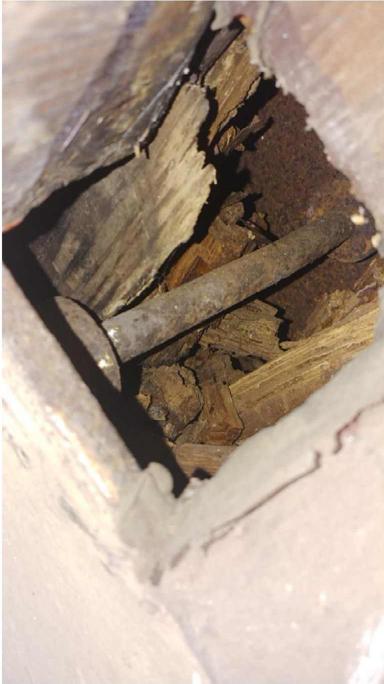
Photo 5 – Exposed \frac{3}{4} " diameter rods between the steel casing sides thru the deteriorated glulam arch.
