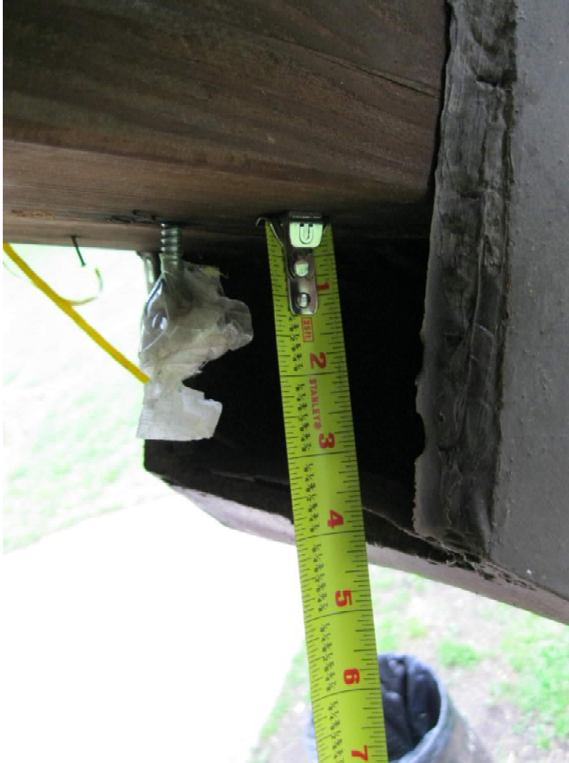
Photo 3 – Separation of the steel casing from glulam arch.
