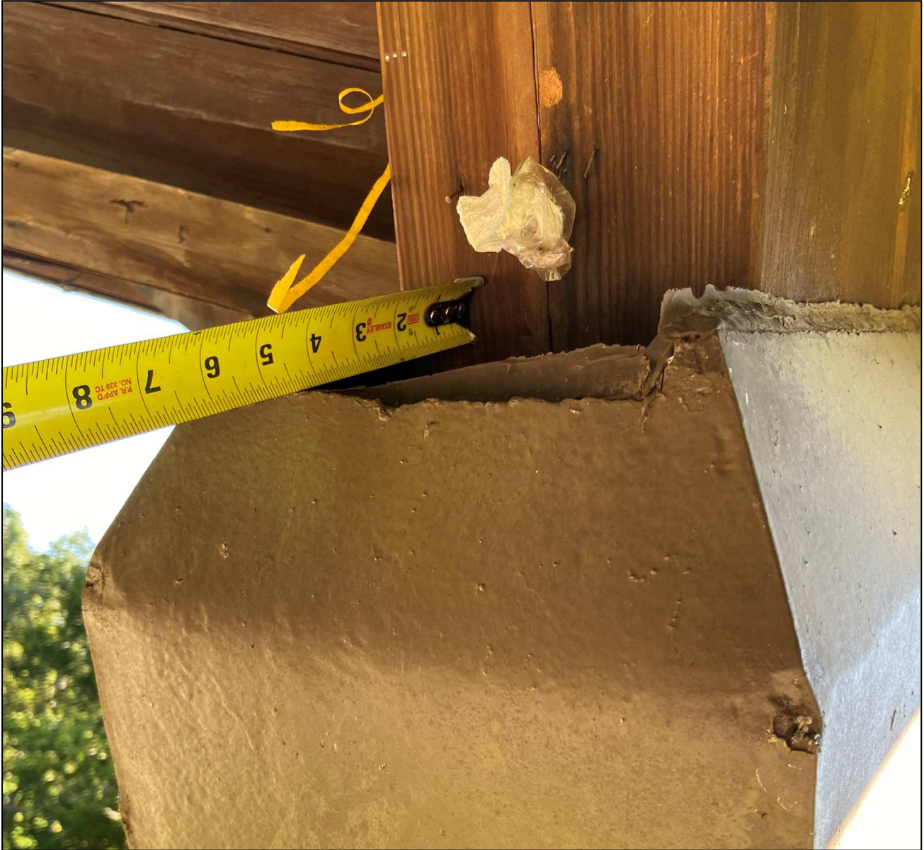
Photo 4: Measured Gap at Beam #6
