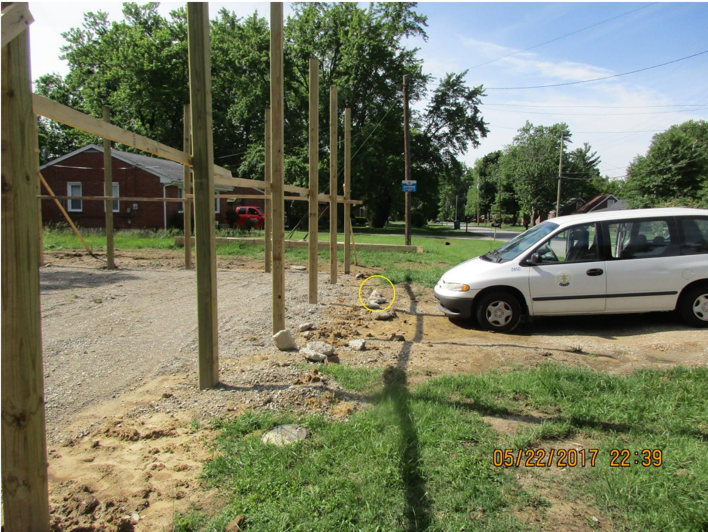
The circled bottle is at the approximate location of the property line.
