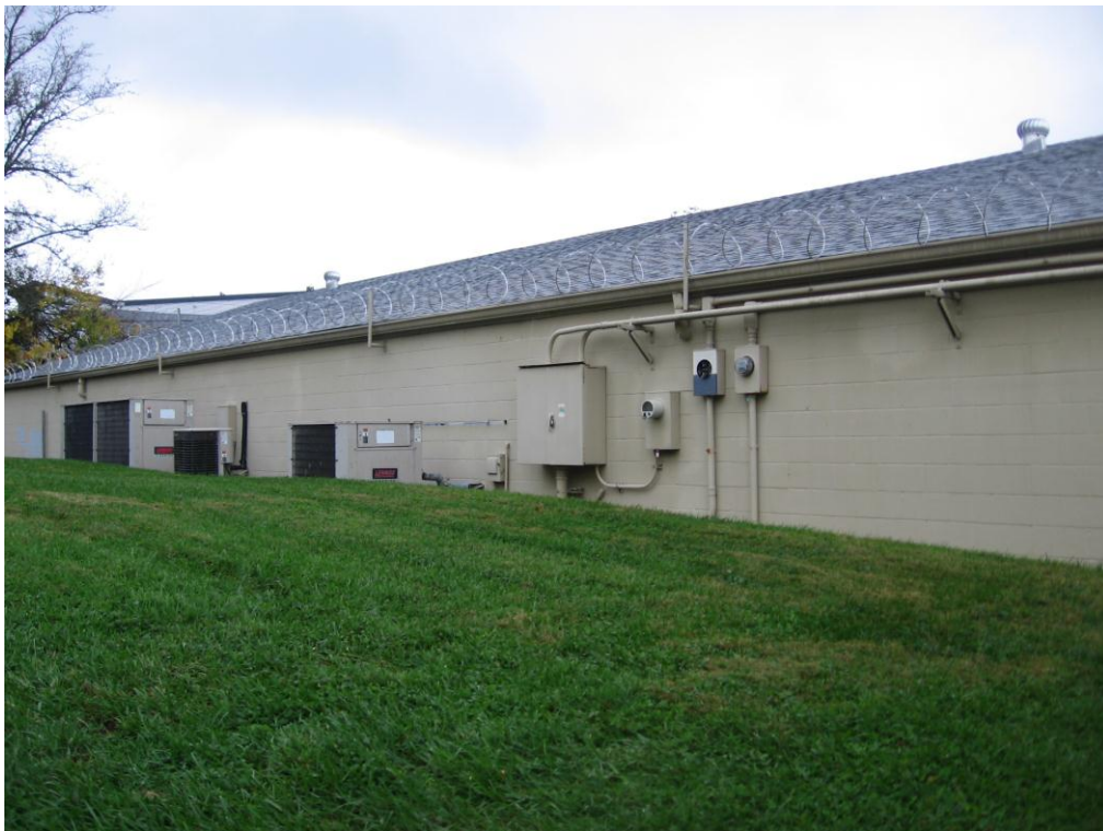
Razor Wire along edge of roof of Alliance Machine Tool Company building next to the vacant lot
