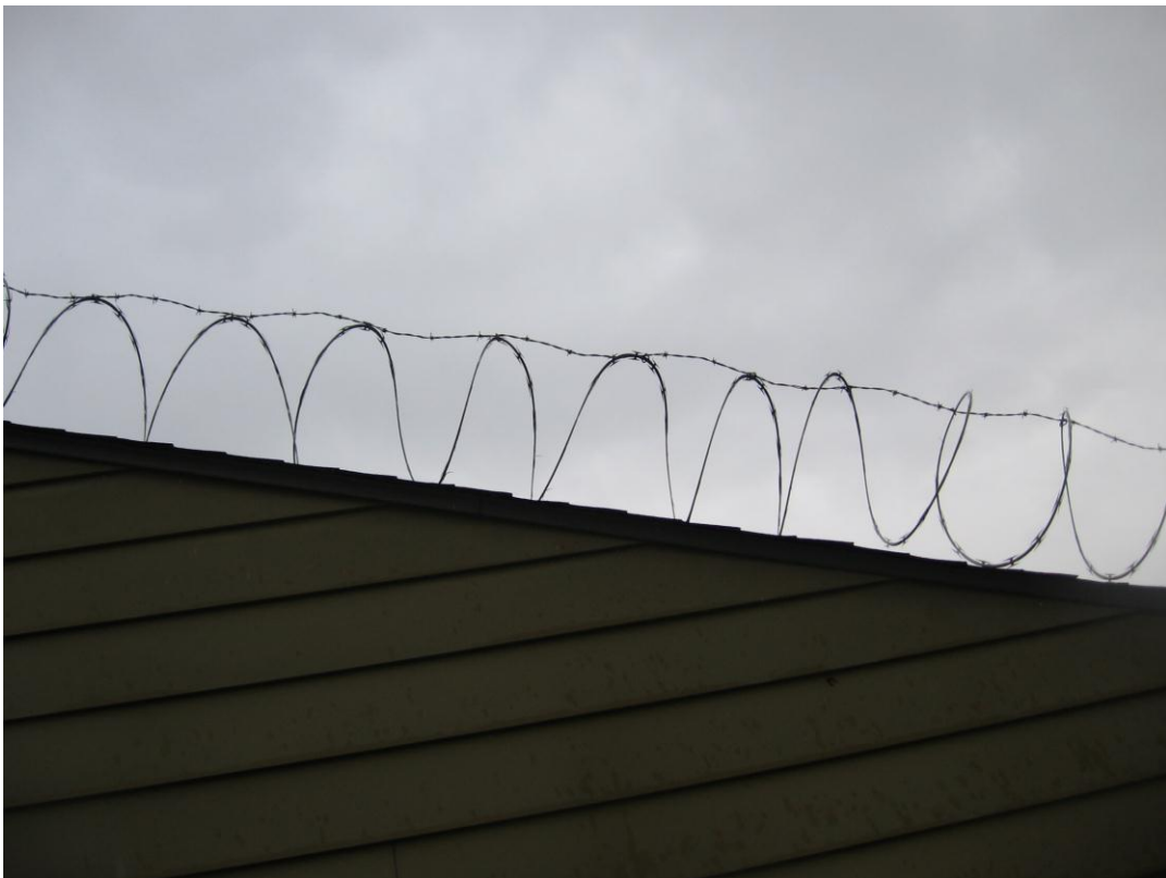
Razor Wire along the edge of the roof of the Alliance Machine Tool Company building
