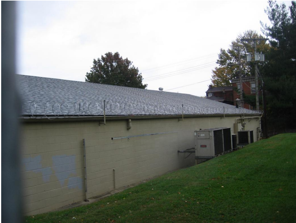
Razor Wire along edge of roof of Alliance Machine Tool Company building next to the vacant lot
