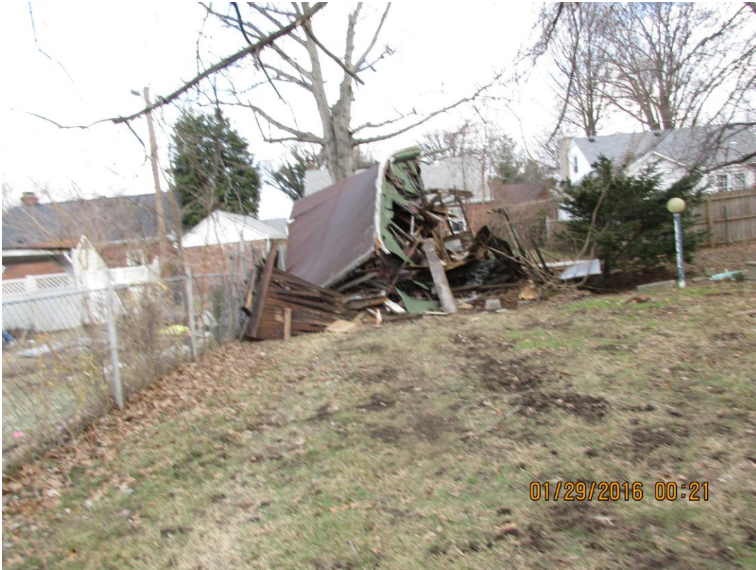
Rear yard of the property looking at a different angle (Looking NE) of the dilapidated garage to be replaced.
