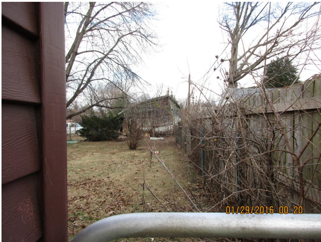
Side Yard looking towards rear of property at the dilapidated garage. (looking NW)
