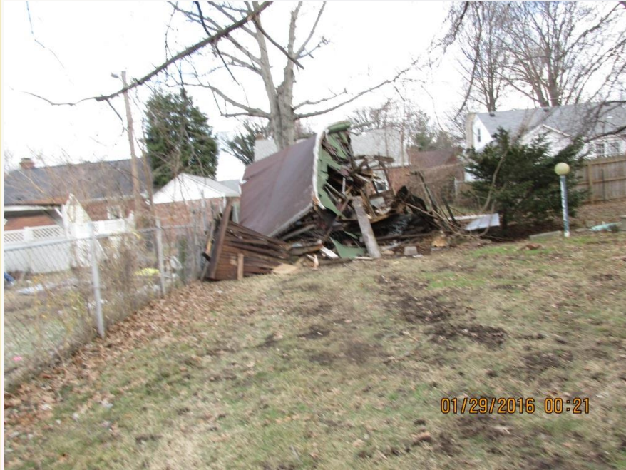
Rear yard of the property looking at a different angle (Looking NE) of the dilapidated garage to be replaced.
